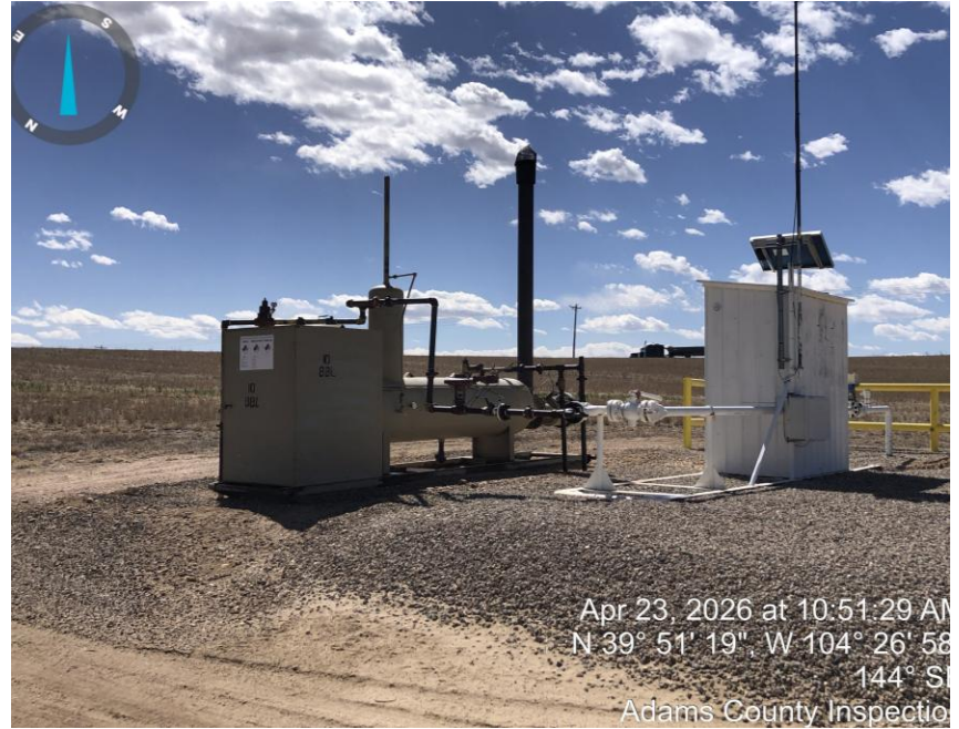
Photo #2 Separator & Meter house.
