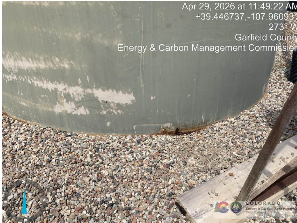
East tank was repaired with a screw. Another seep has shown up within inches of the last seep.
