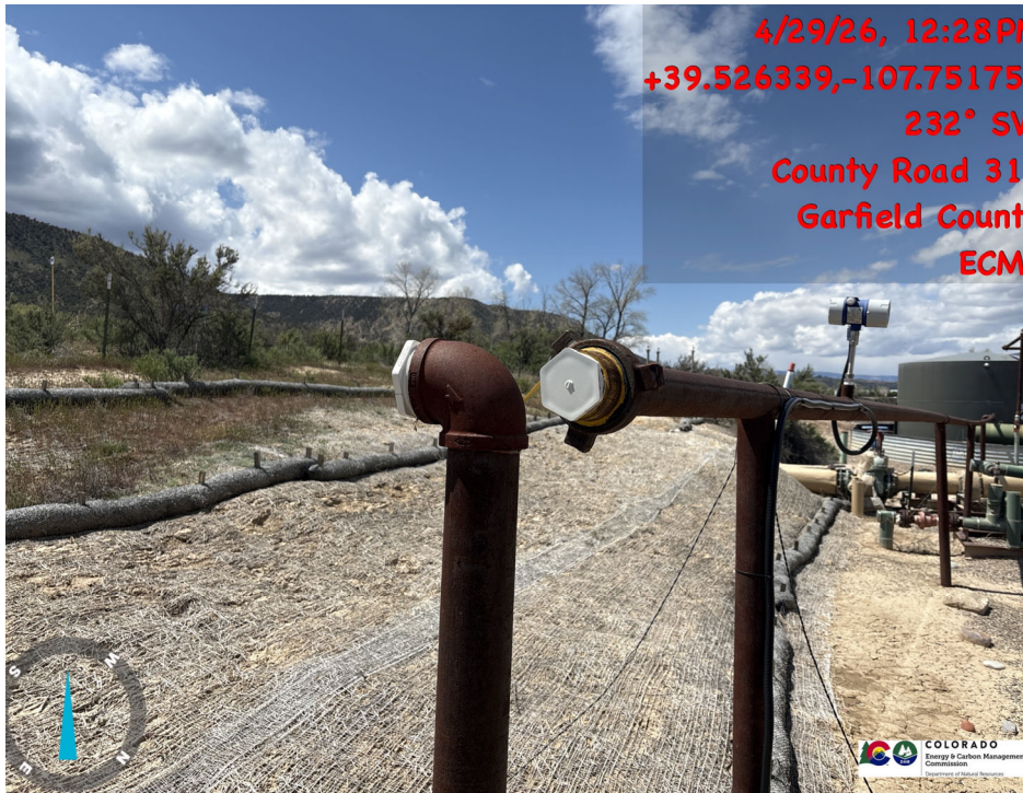
Main line for ECD is disconnected
