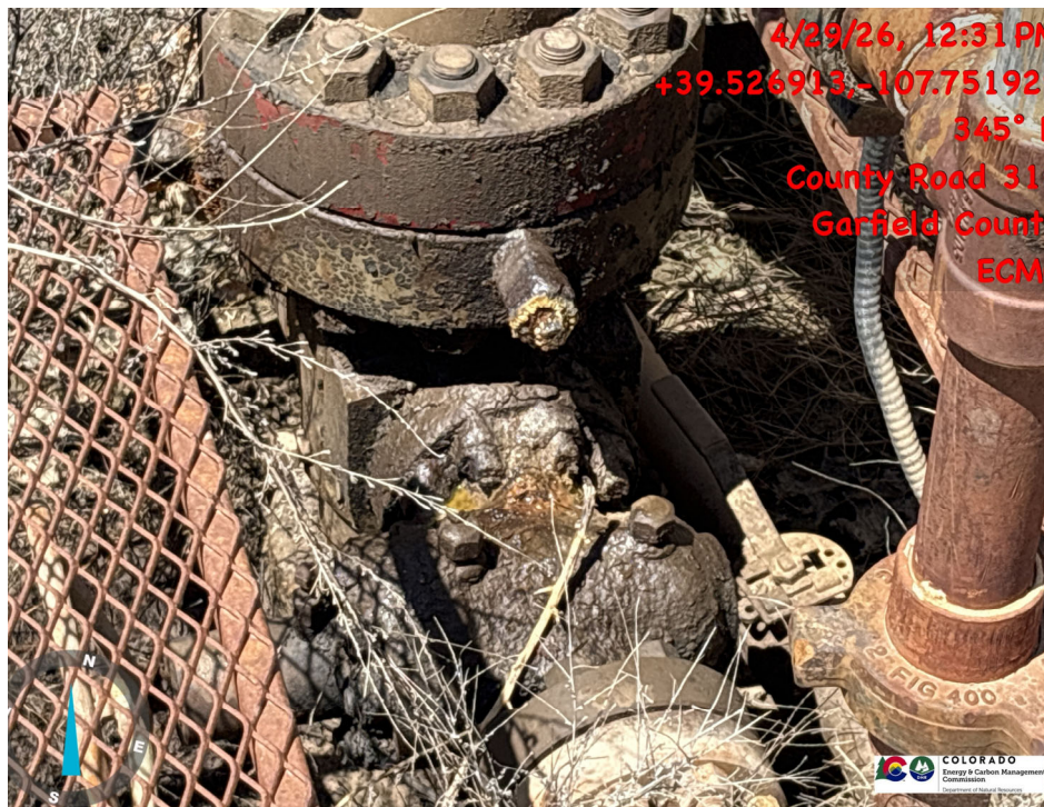
Well head leaking
