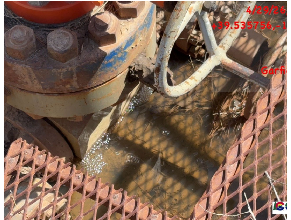
Well head leaking (bubbling)
