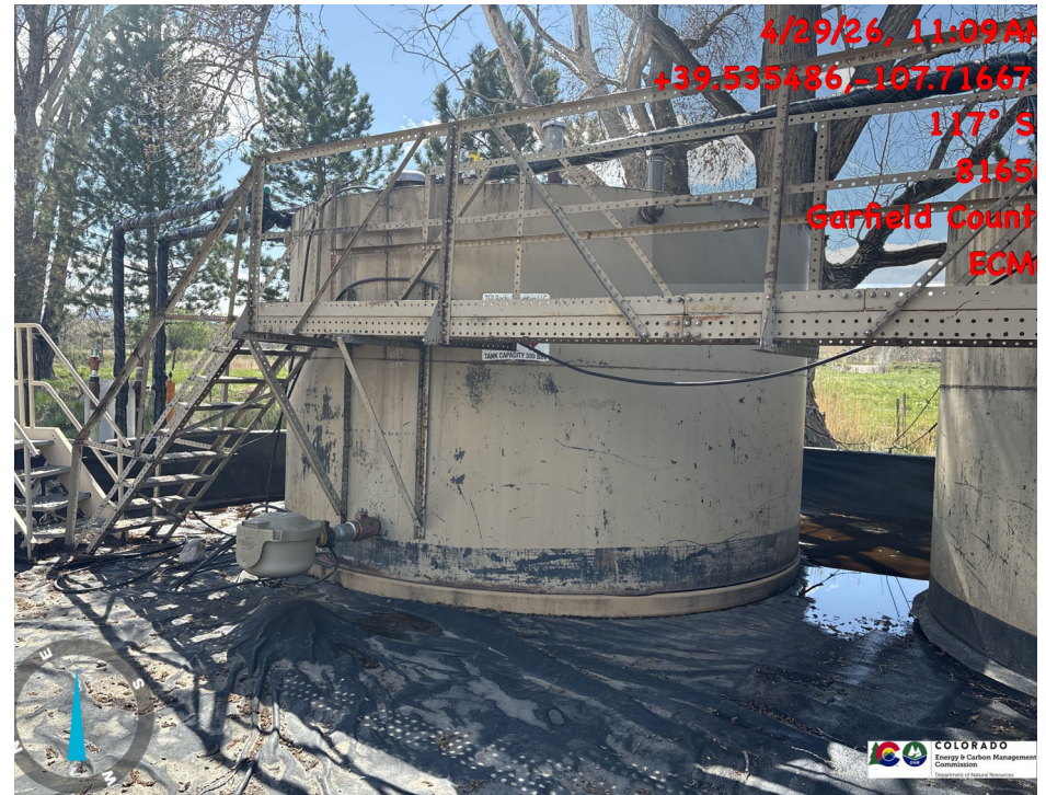
Tank labeling is not visible from a distance
