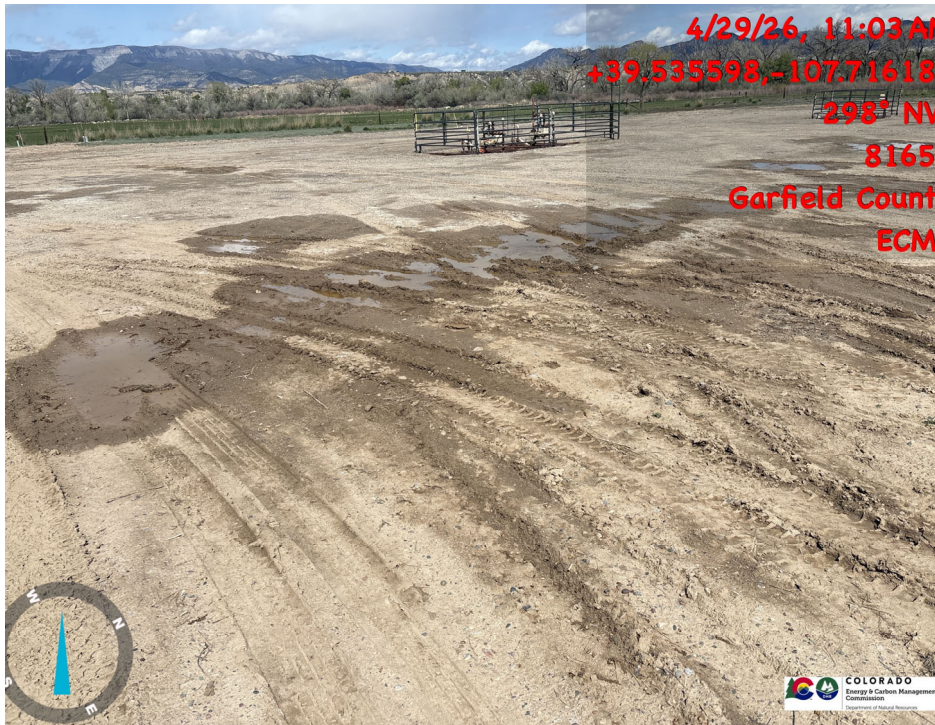
Some areas of location show signs of lack of stabilization/compaction
