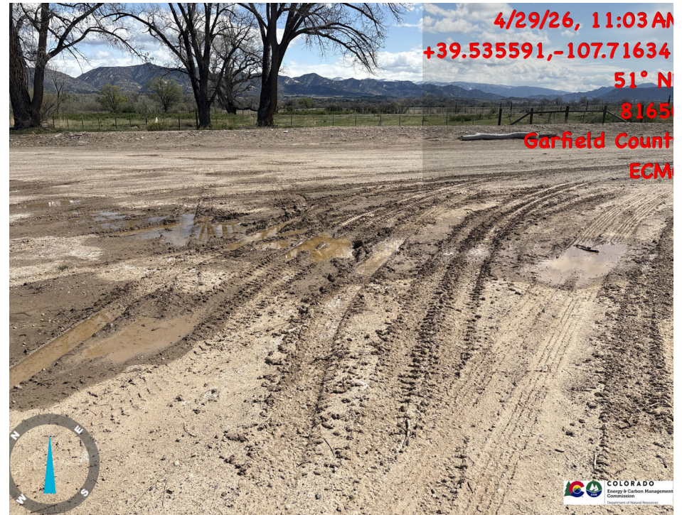
Some areas of location show signs of lack of stabilization/compaction
