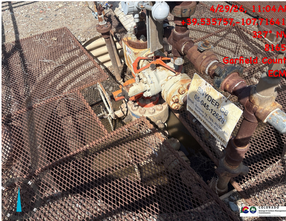
Well head leaking (bubbling)
