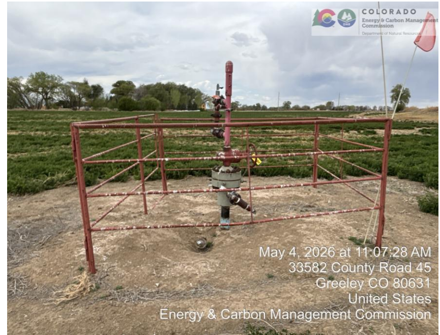
Photo 2 well head and equipment
