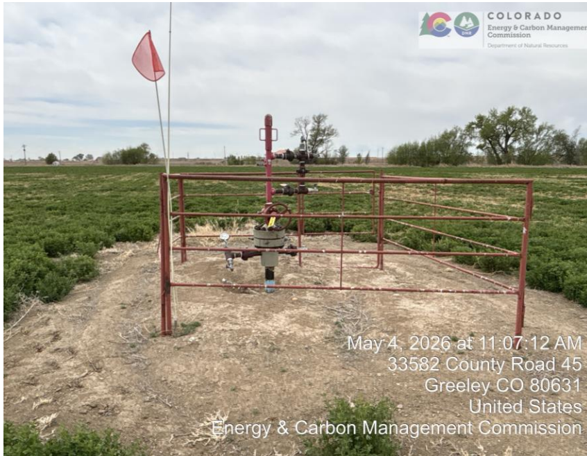
Photo 1 well head and equipment
