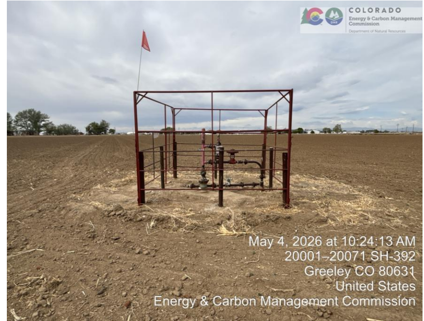
Photo 2 well head and equipment
