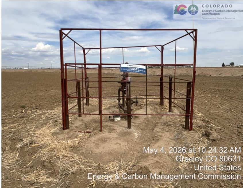
Photo 1 well head and equipment
