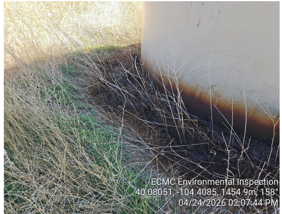
Photo 6 – Spill observed around AST
