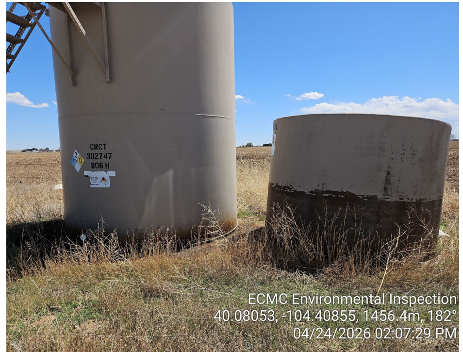
Photo 2 – Spill observed around AST
