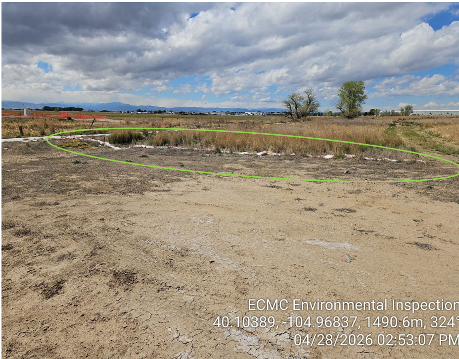
Photo 7 – Stormwater waddles have degraded and become trash (green).
