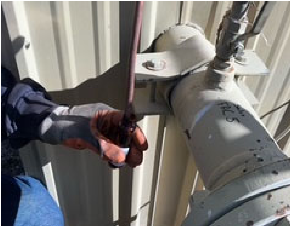
Attempted condensate sampling from Facility 5 Gas Sales Line – No condensate produced
