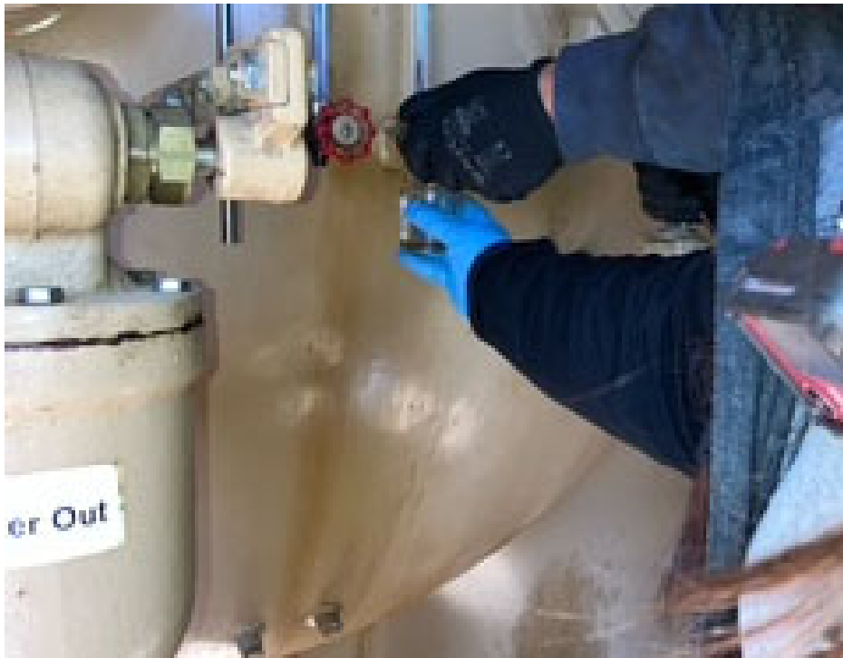
Oil Sampling from Facility 5 Horizontal Separator Oil Sight Glass
