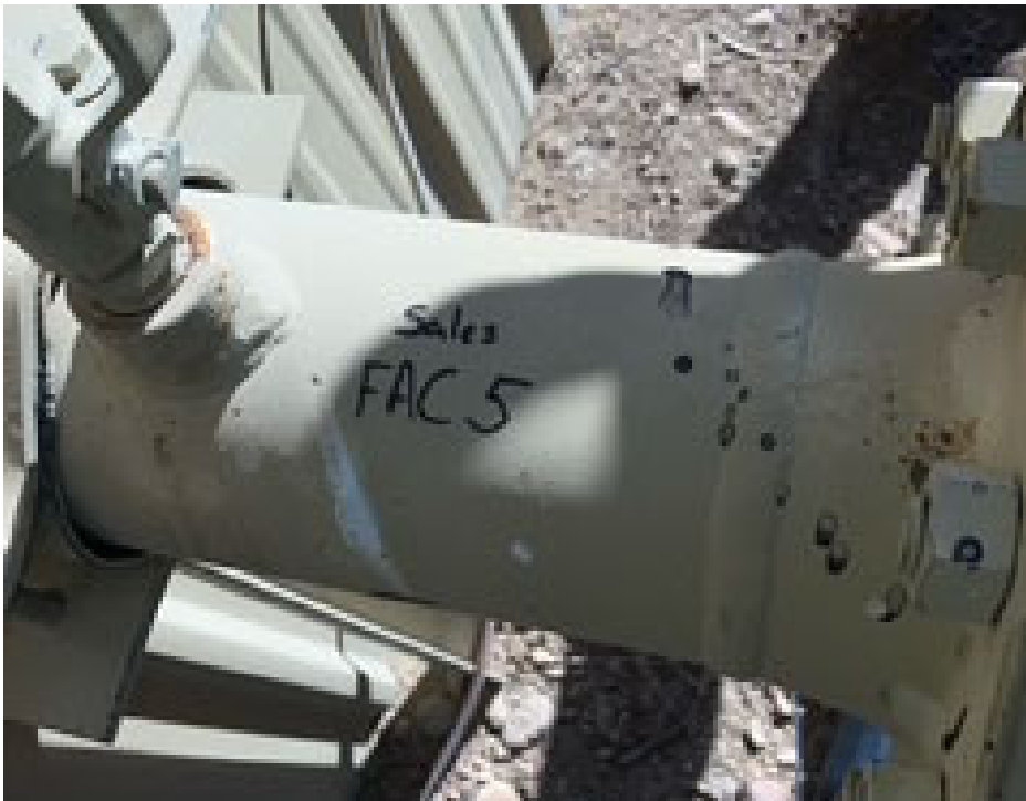
Facility 5 Gas Sales line
