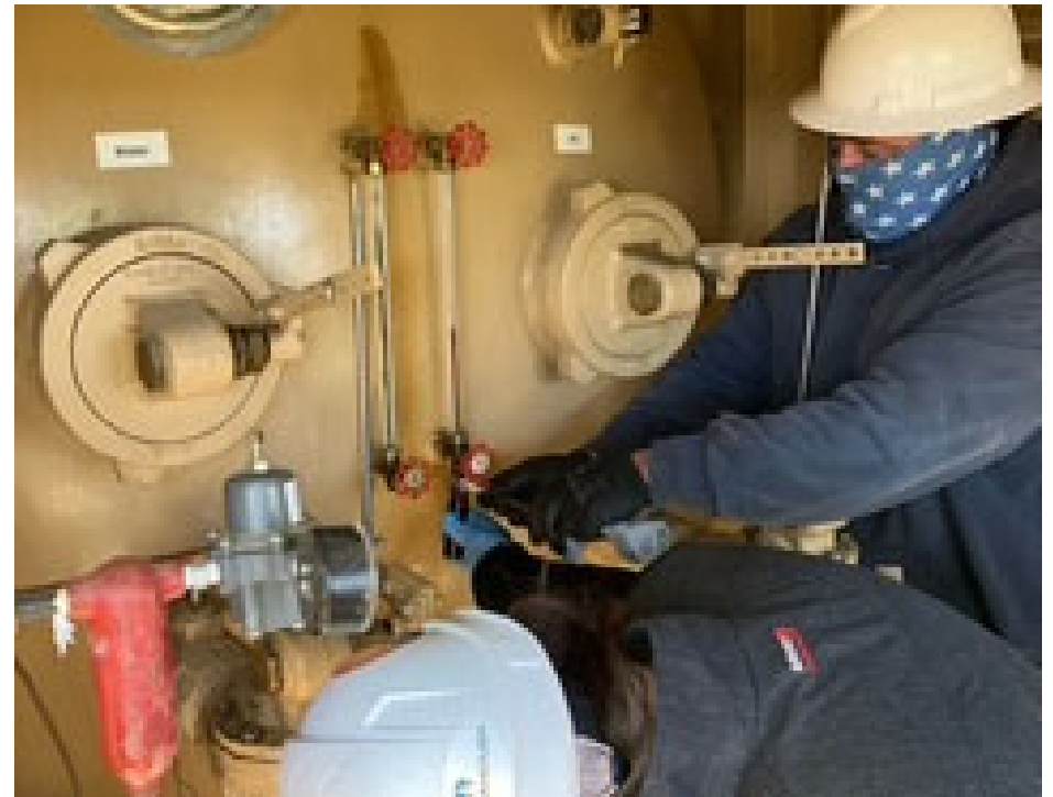
Oil Sampling from Facility 5 Horizontal Separator Oil Sight Glass
