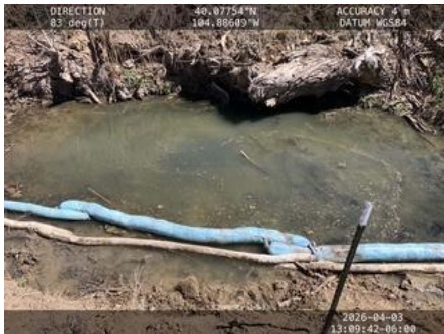
Hydrophobic oil-absorbent booms installed within Little Dry Creek adjacent to former excavation.
