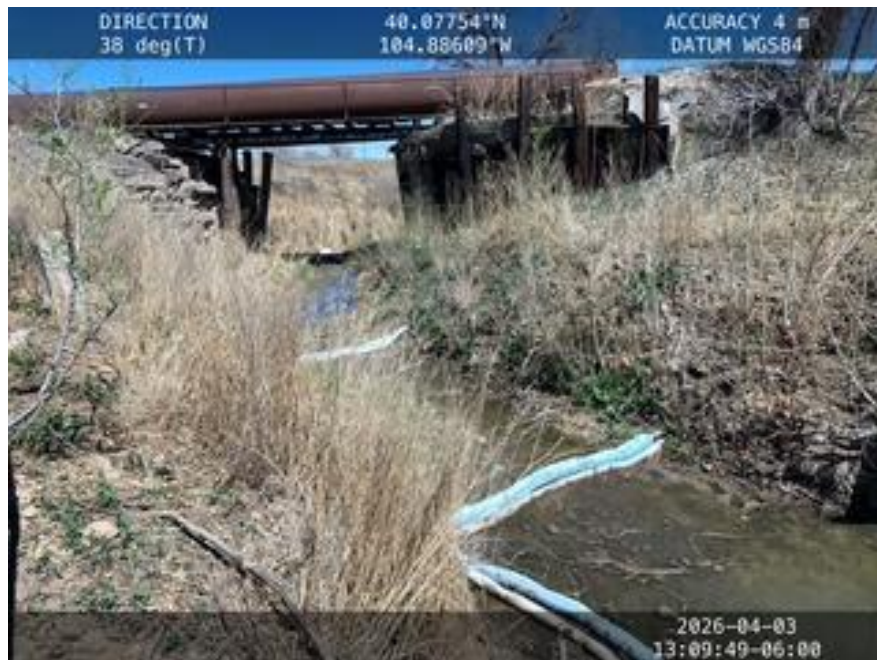
Hydrophobic oil-absorbent booms installed within Little Dry Creek downstream of former excavation.
