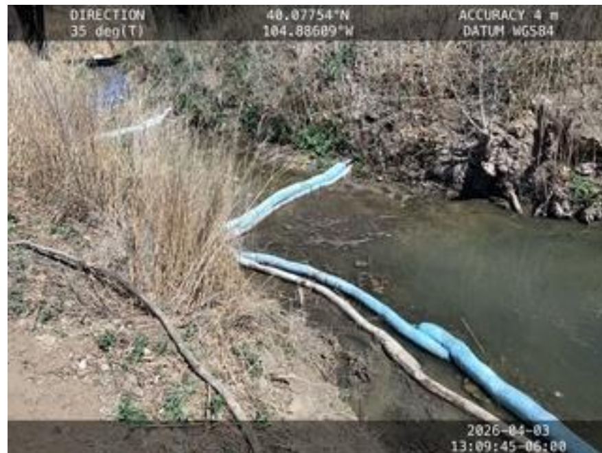
Hydrophobic oil-absorbent booms installed within Little Dry Creek adjacent to former excavation.
