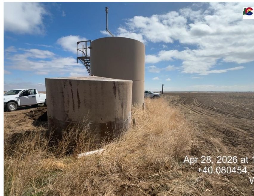
Pic 16 weeds unmanaged, berms not adequate.
