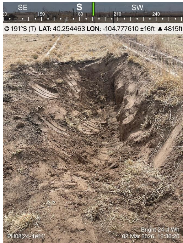
Flowline Pothole Screening Location 09 (Photo Mislabeled)
