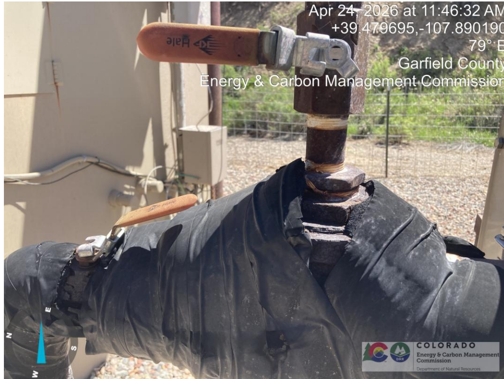
Rusted valves and fittings on catalytic heater.
