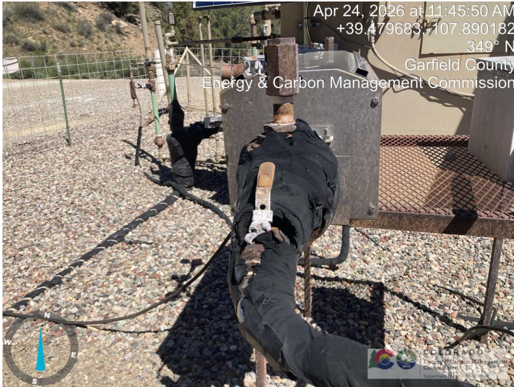
Rusted valves and fittings on catalytic heater.
