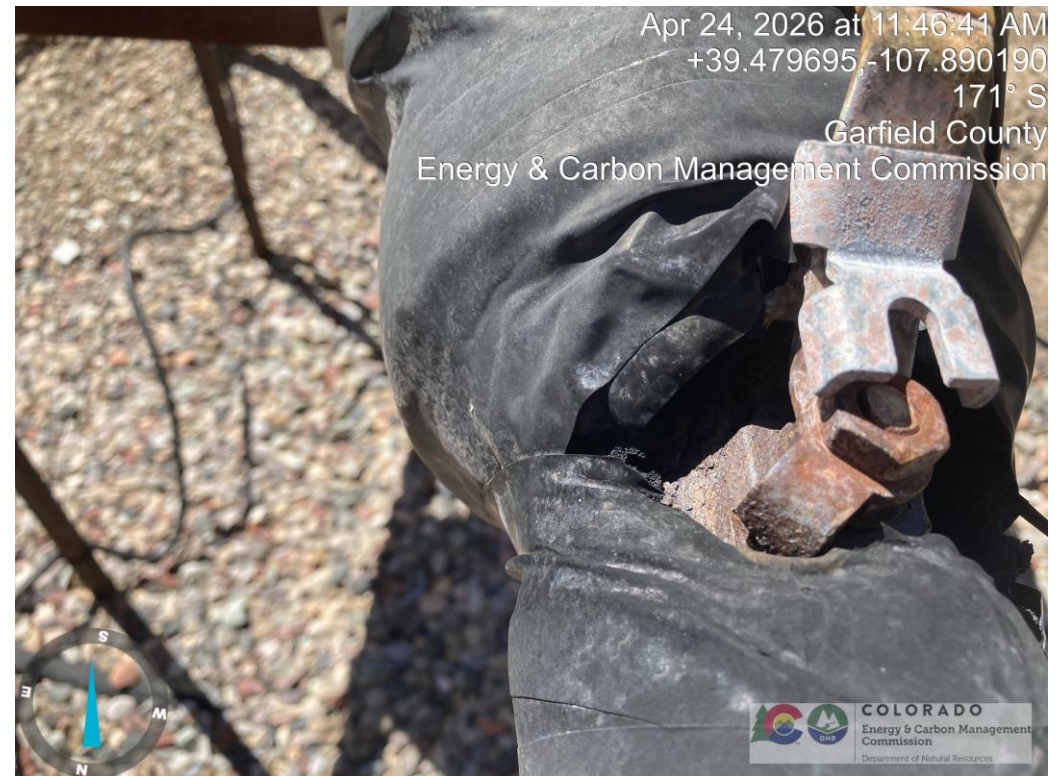
Rusted valves and fittings on catalytic heater.
