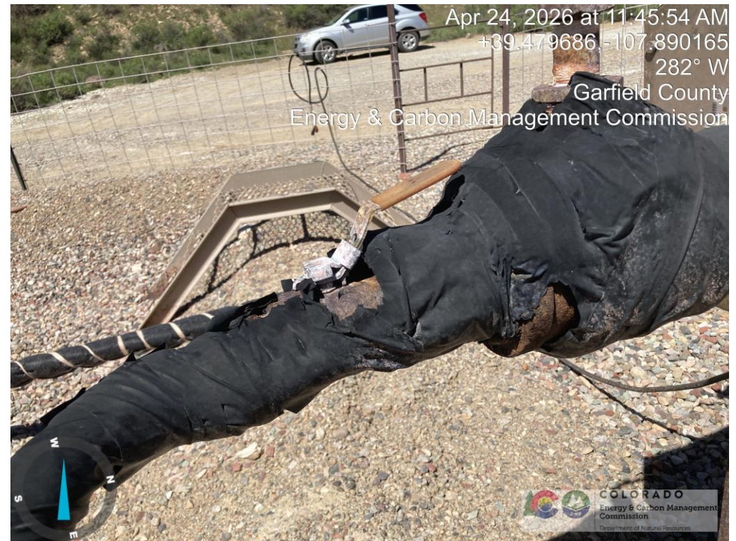
Rusted valves and fittings on catalytic heater.
