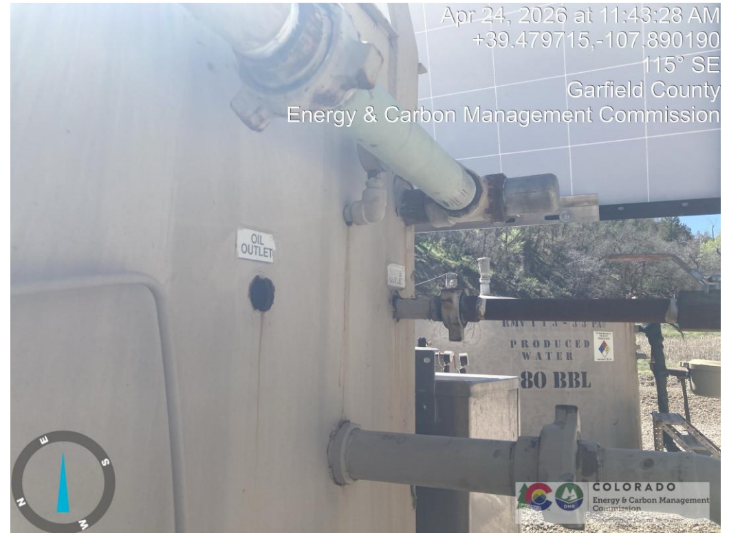
Unpainted and/or Paint deterioration and areas of rust.
