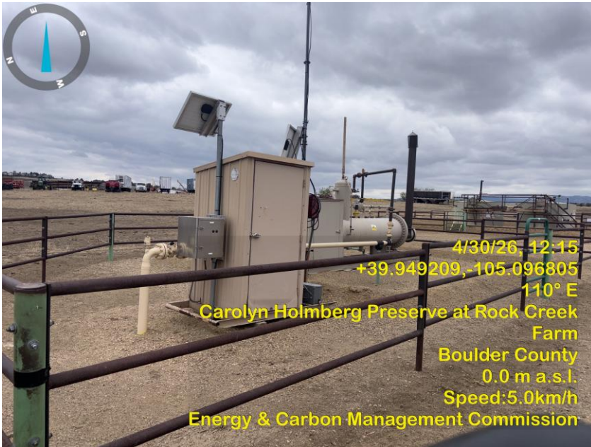
Photo 3 Gas meter run.
