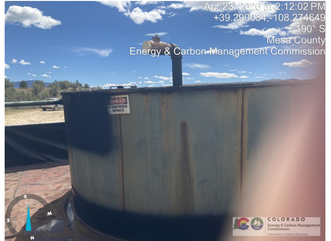
Seep hole on side of tank.
