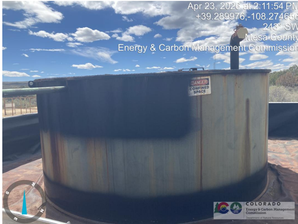
Seep hole on side of tank.
