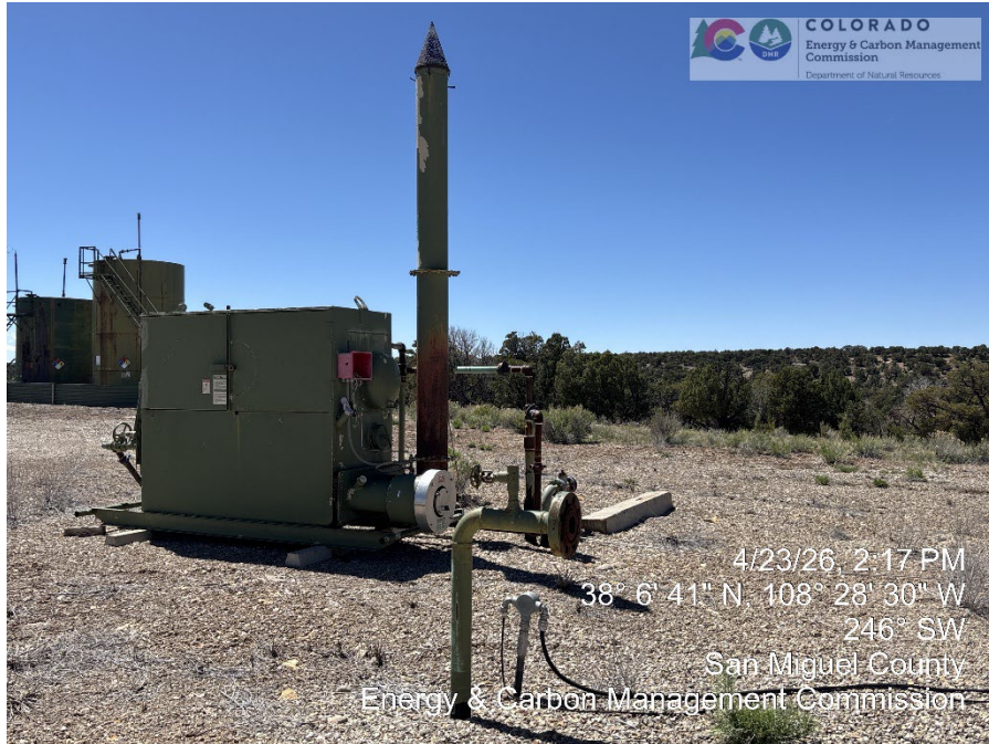
Open ended flowline at separator
