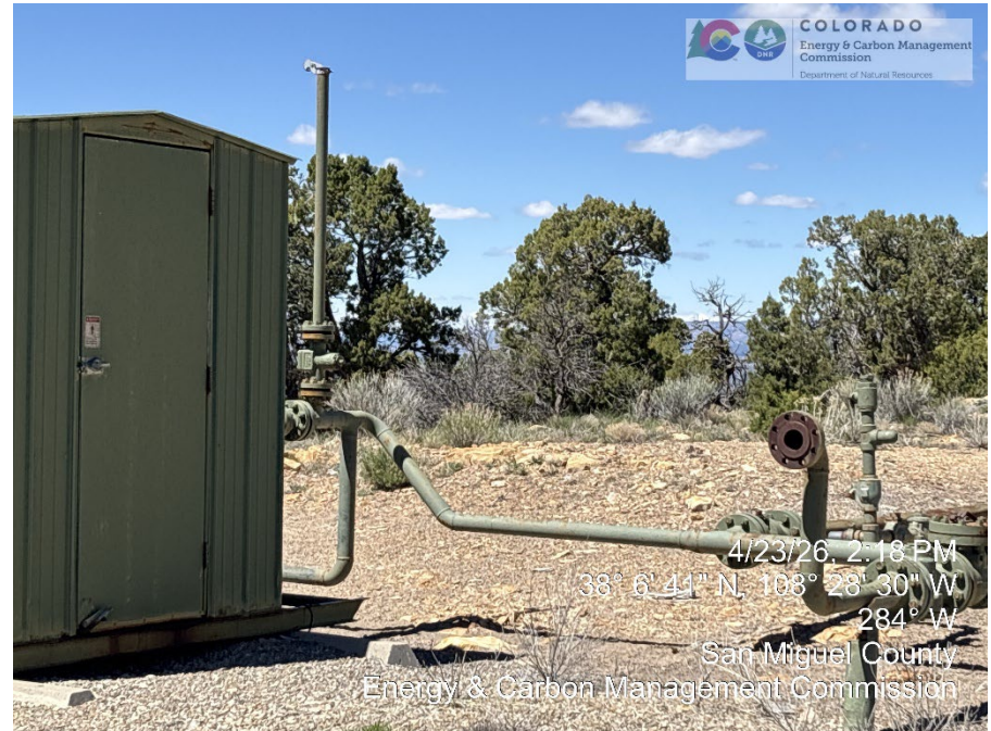
Open ended flowline at meter housing
