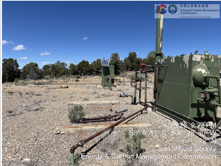
Separator and Meter housing Disconnected and blind flanged
