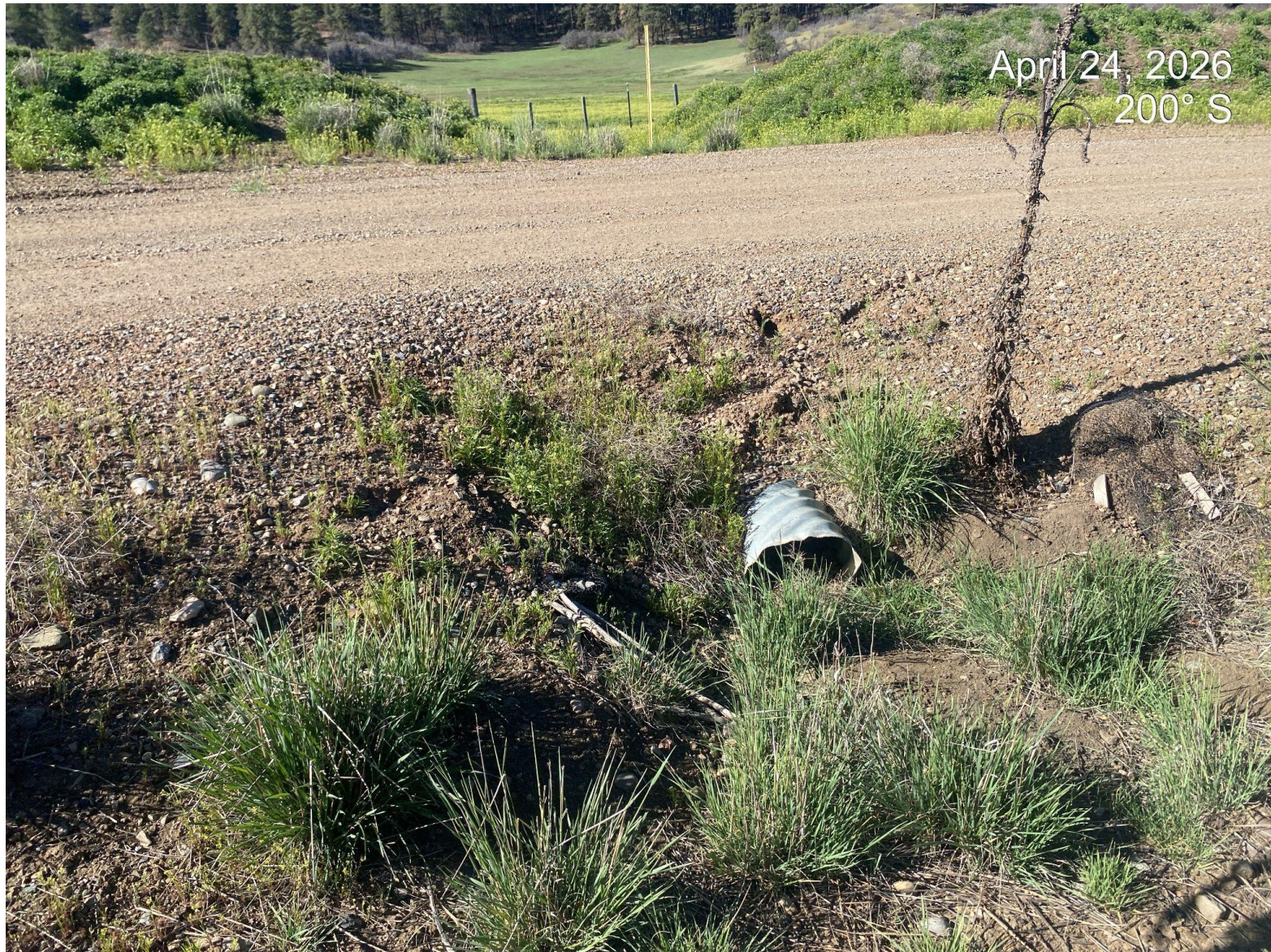
Photo 3. Culvert at access point is starting to fill with sediment.
