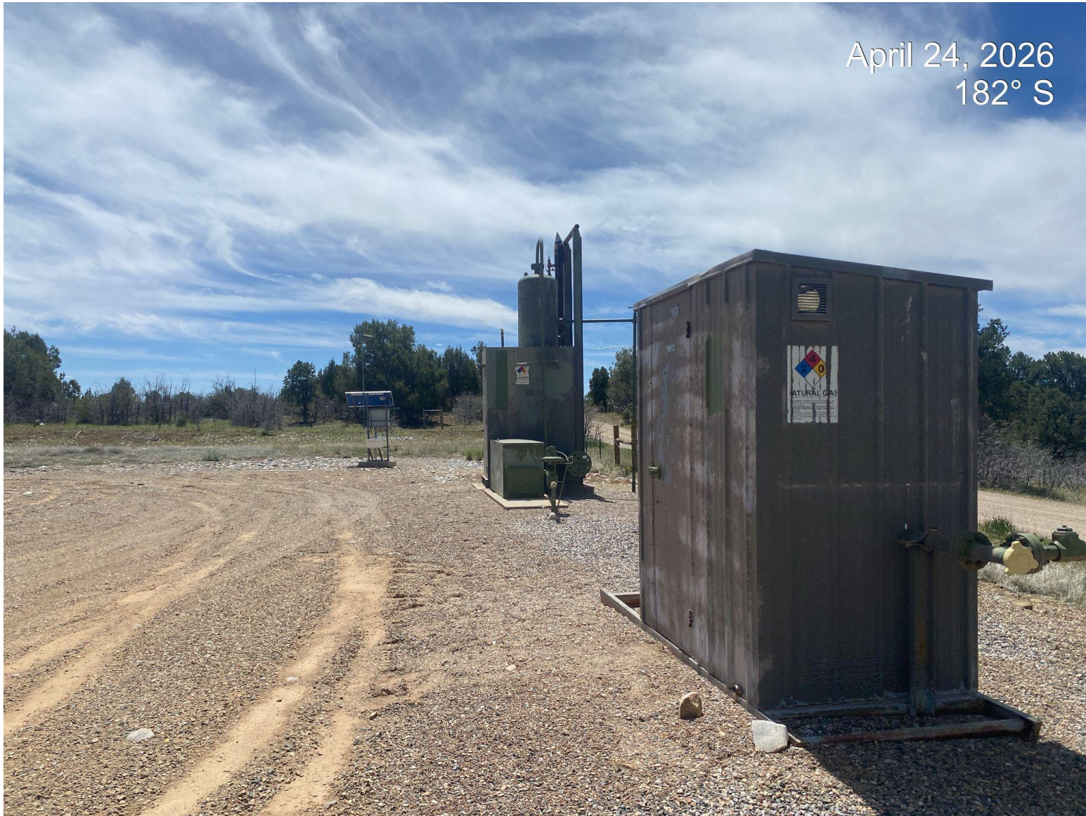
Photo 2. View of meter shed and separator equipment, labels are starting to deteriorate/peel.
