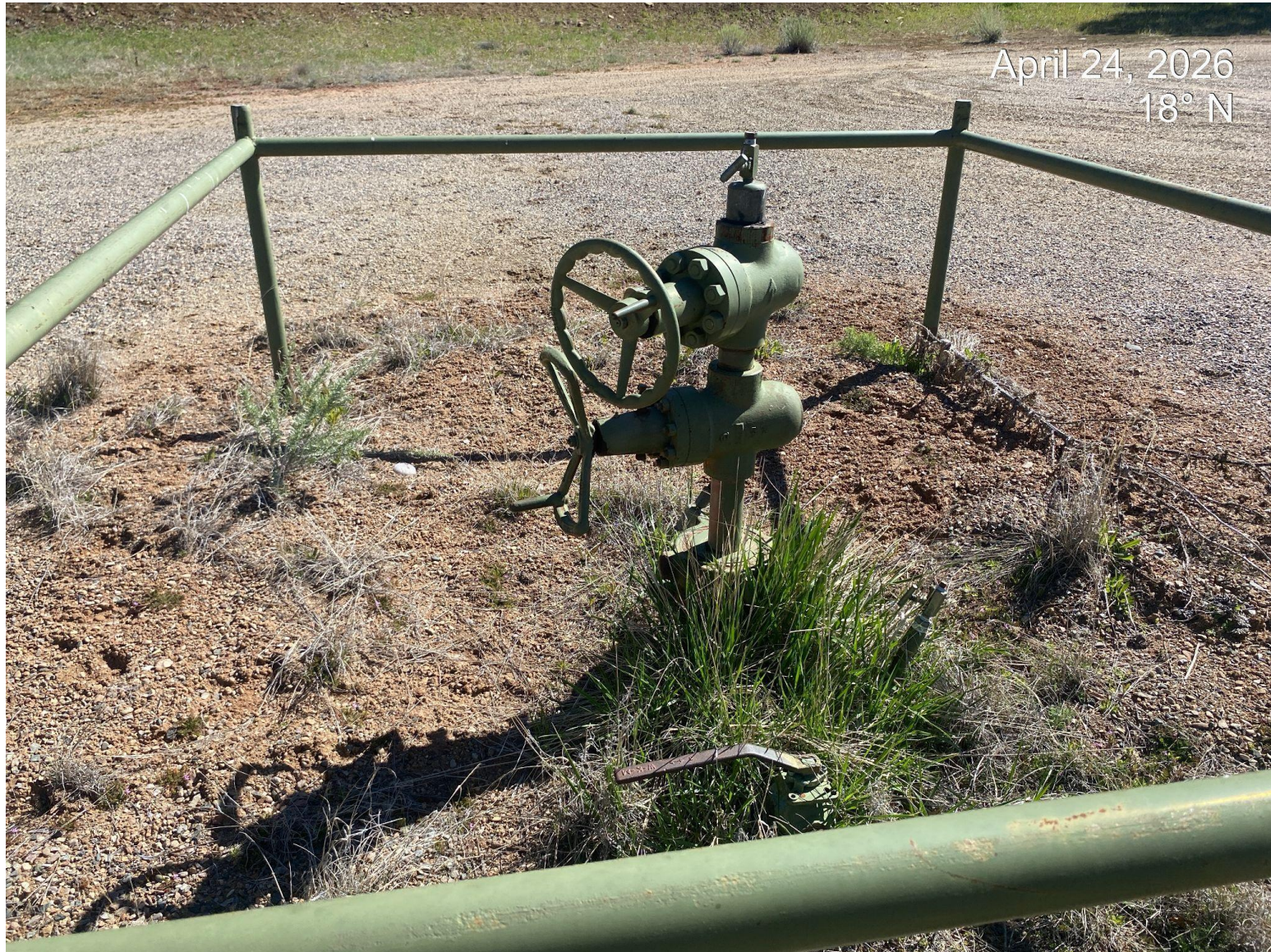
Photo 3. Wellhead assembly equipment; vegetation encroaching on equipment.
