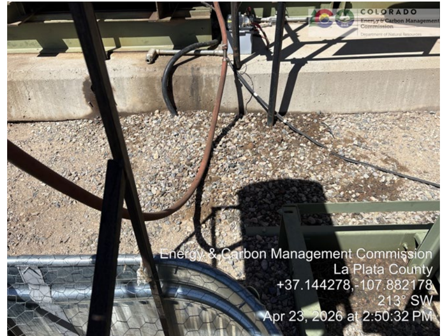
14. After. Gravel sprinkled over top, not cleaned up, leak does not appear to be repaired.
