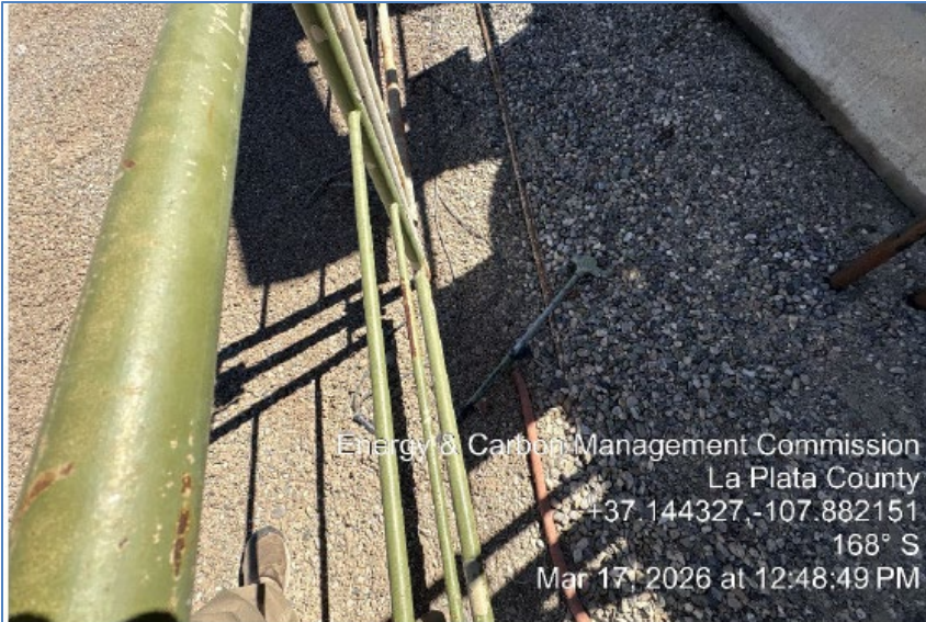
40. Conduit and loose wire at 36-1A.
