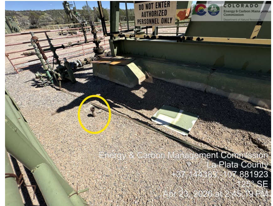
46. Unmarked out of service riser remains.
