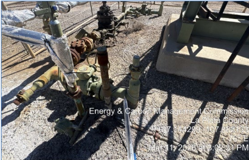
18. 36-2A Wellhead area pen indicates wires, some of which appear to be frayed. There is dead vegetative debris near the wellhead
