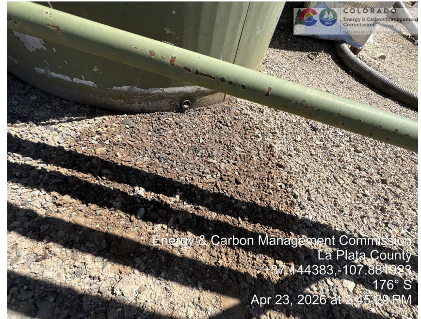
44. After. Drain plug remains missing. Soil remains stained.
