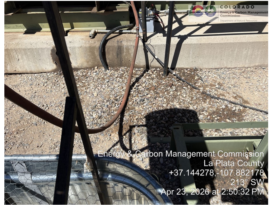
10. After. Gravel has been sprinkled over top of stained material but not cleaned up. Different angle.
