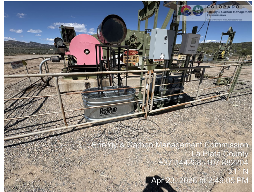
28. After. Wires remain on ground.
