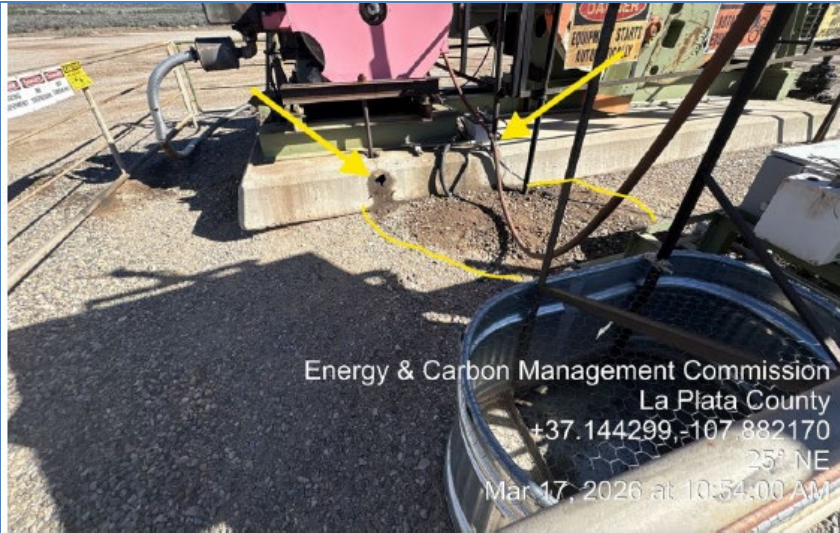
33. Lube tank hose leak and prime mover drain leak in foundation.
