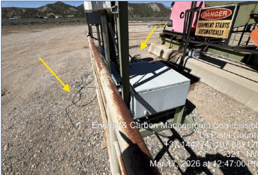
41. Loose/frayed wire at 36-2A telemetry.
