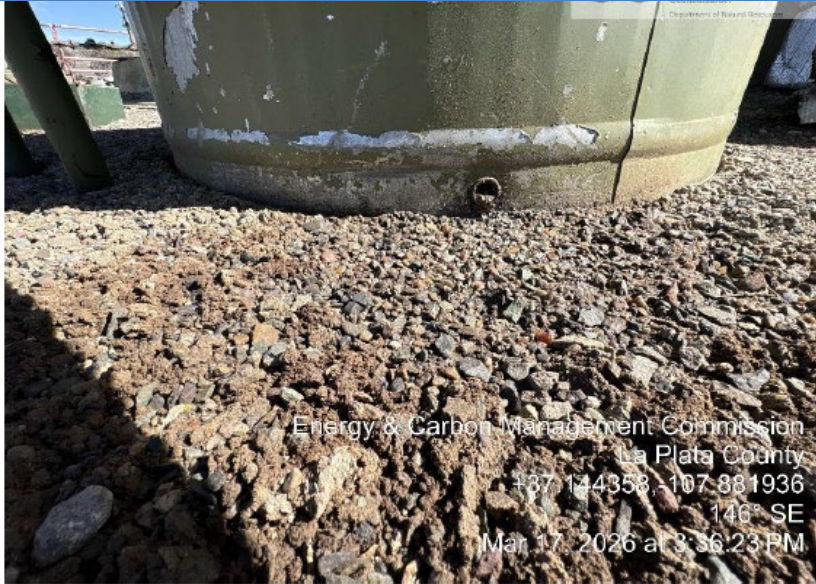
39. Drain plug missing from lube oil tank at 36-1A
