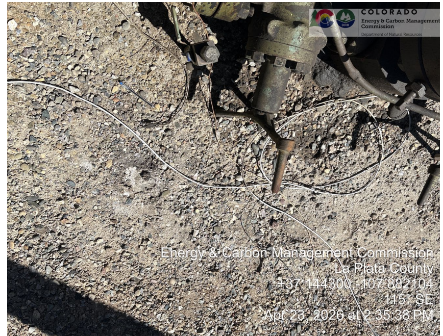
24. After. Different angle. Wires remain on ground.
