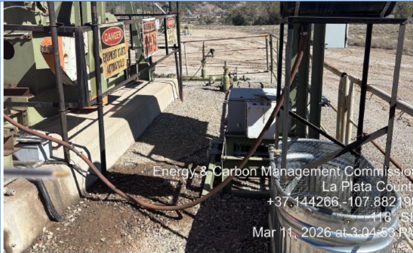
19. 36-2A lube oil tank above secondary containment. The gravity fed hose from the lube tank appears to be leaking and staining the ground, possibly from the location where two segments of hose are connected with a pipe nipple and two hose clamps.
