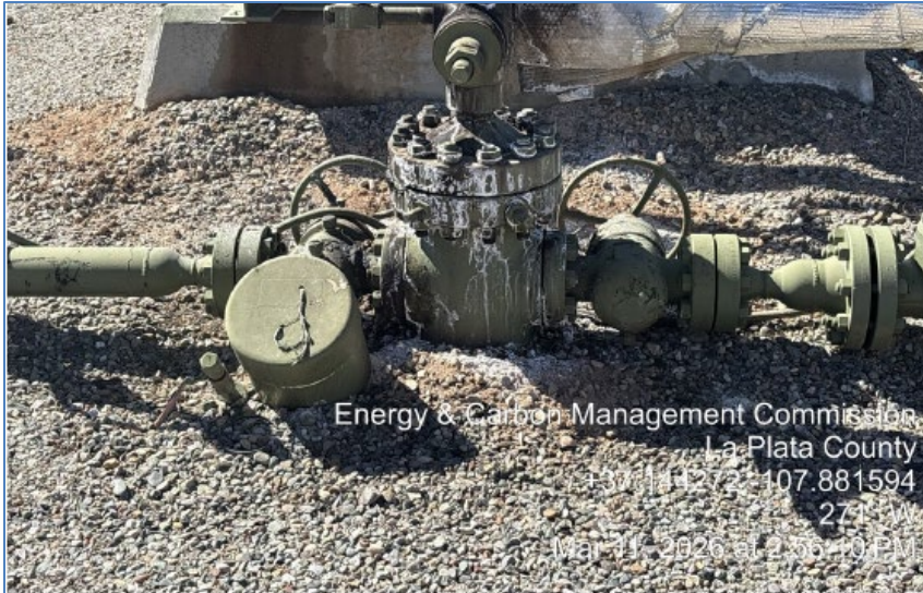
7. 36-1 wellhead. White mineralization appears to be salt residue from produced water seepage.
