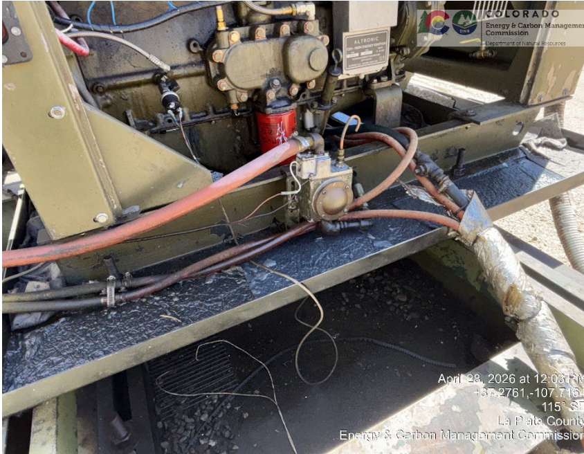
ENGINE SKID LEAK
