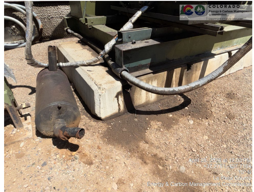
ENGINE SKID LEAK
