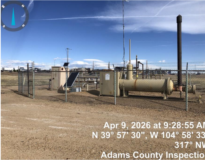
PHOTO#1 GAS METER/AUTOMATION RTU/SEPARATOR
