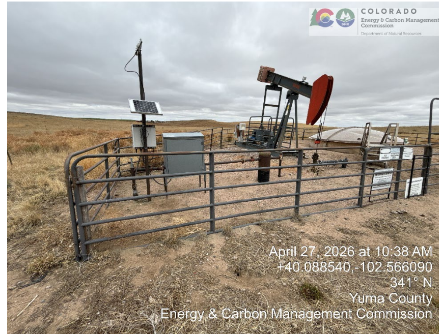
Meter run, PU, and Wellhead
