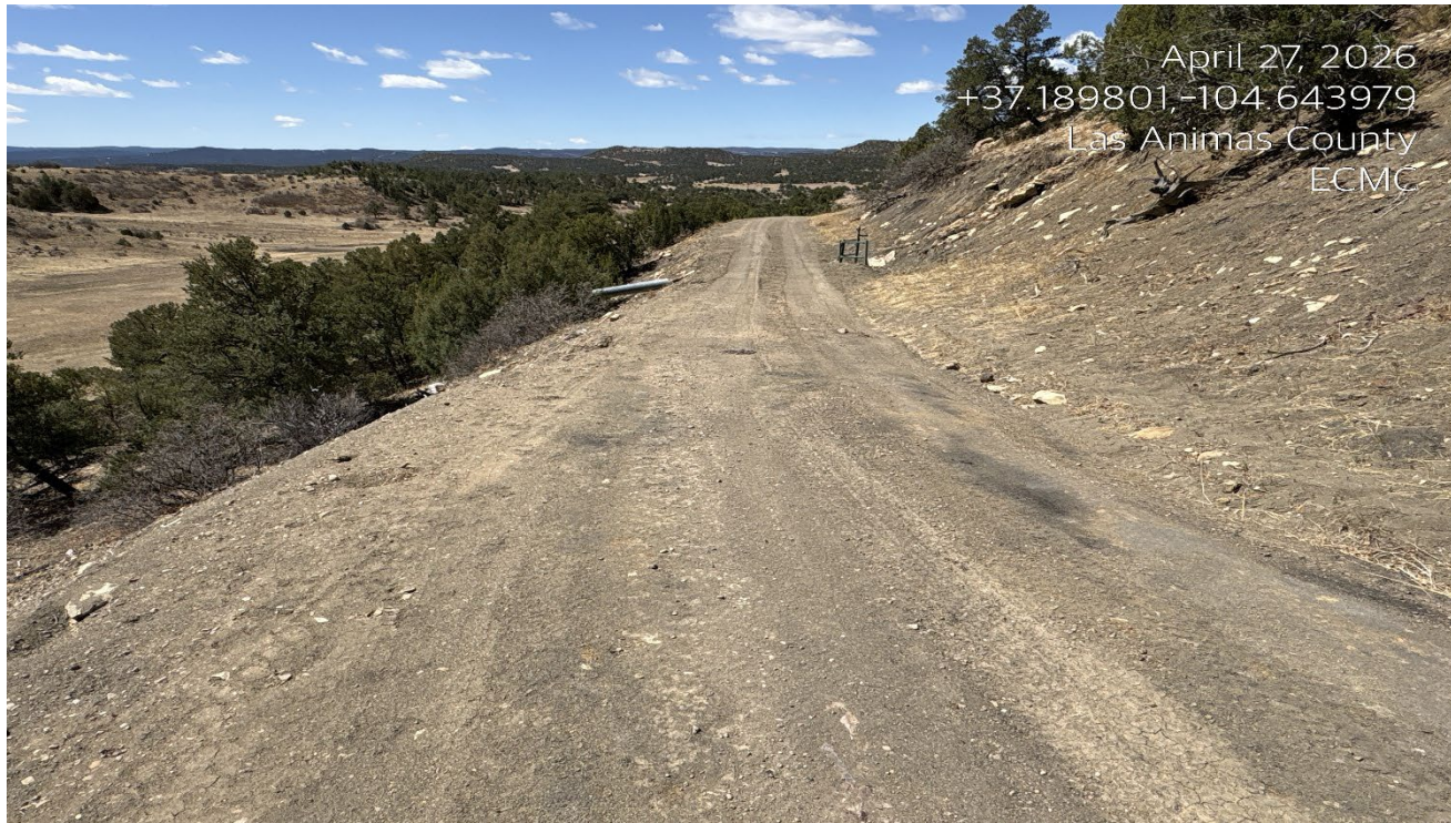
Photo 1. Facing southeast along the access road. The ae of erosion has been repaired and culvert maintained.
