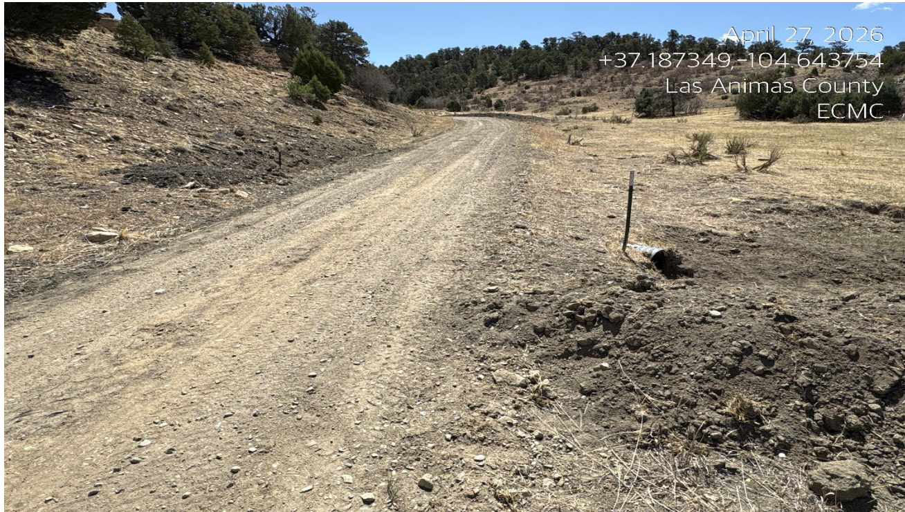
Photo 2. Facing east along the access road. This culvert has been cleaned out.
