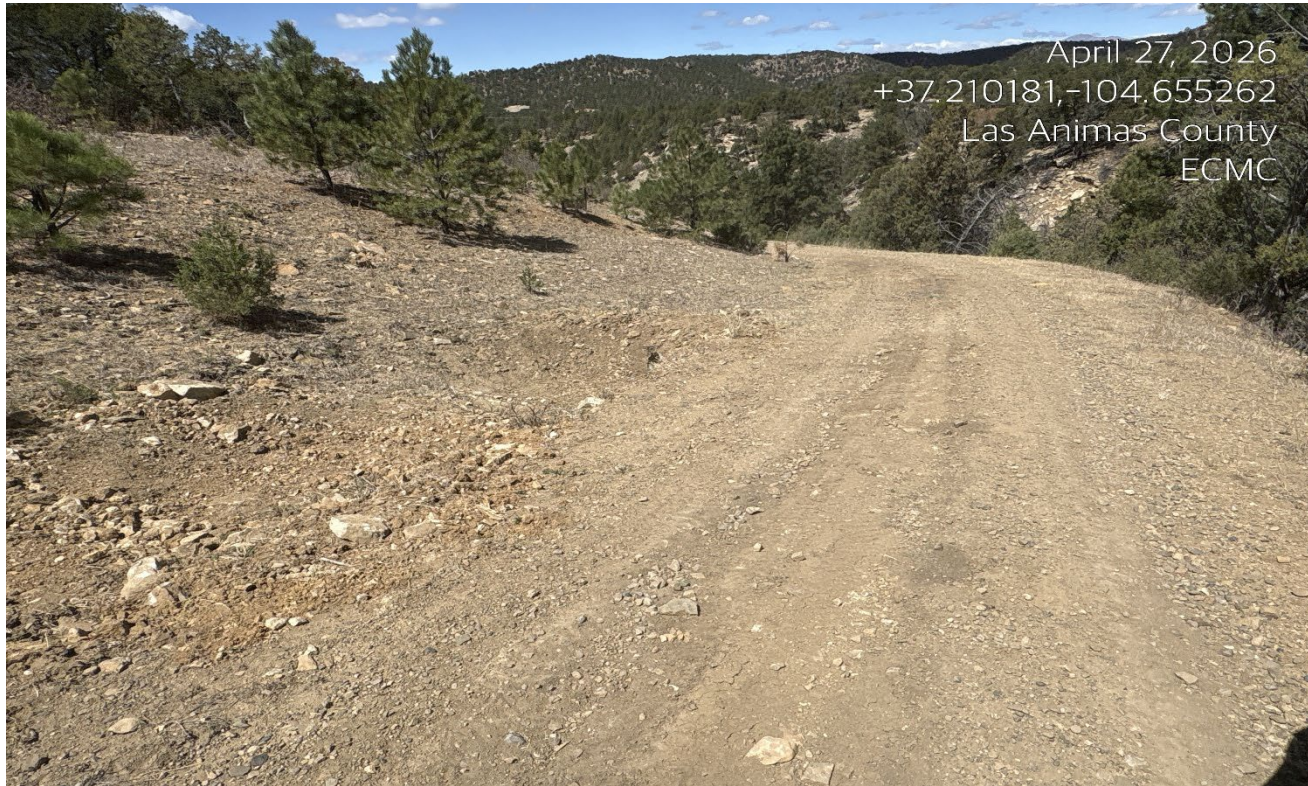
Photo 2. Facing west along the access road. The culverts are cleaned out and maintained.
