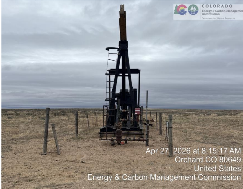
Photo 1 well head and equipment
