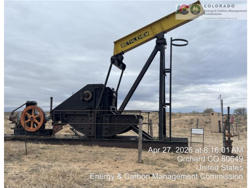
Photo 2 well head and equipment
