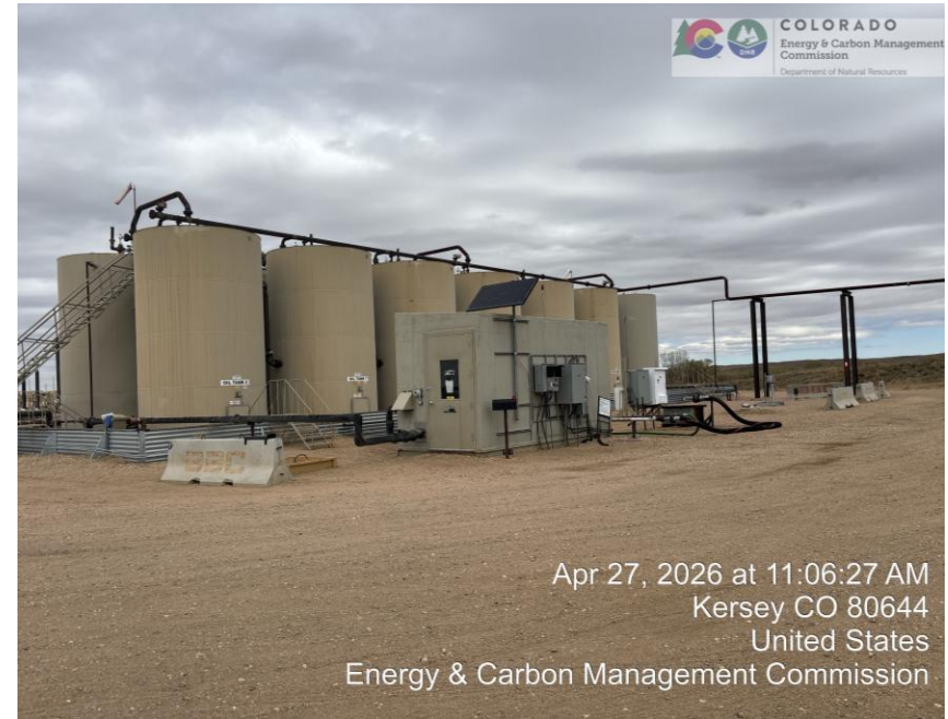
Photo 8 tank battery and equipment
