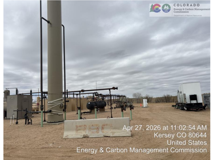
Photo 4 facility and production equipment
