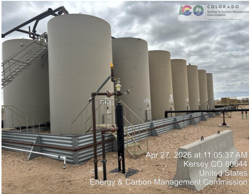
Photo 7 tank battery and equipment
