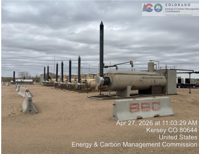
Photo 3 facility and production equipment
