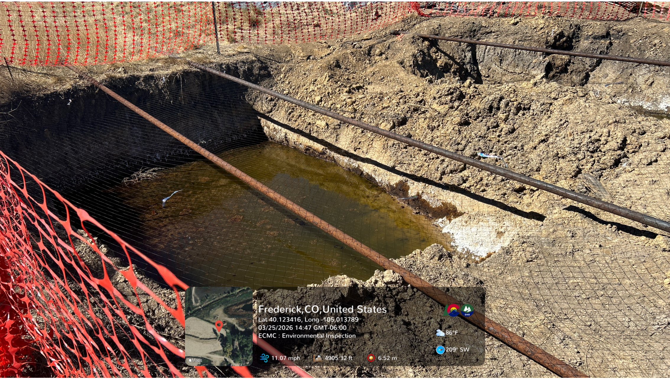
Looking at the southern excavation open at the spill location. Petroleum hydrocarbon saturated soil and salt crusting are visible on the excavation sidewalls. Free product is visible on groundwater at the base of the excavation. Bird netting has been installed over the open excavations.
