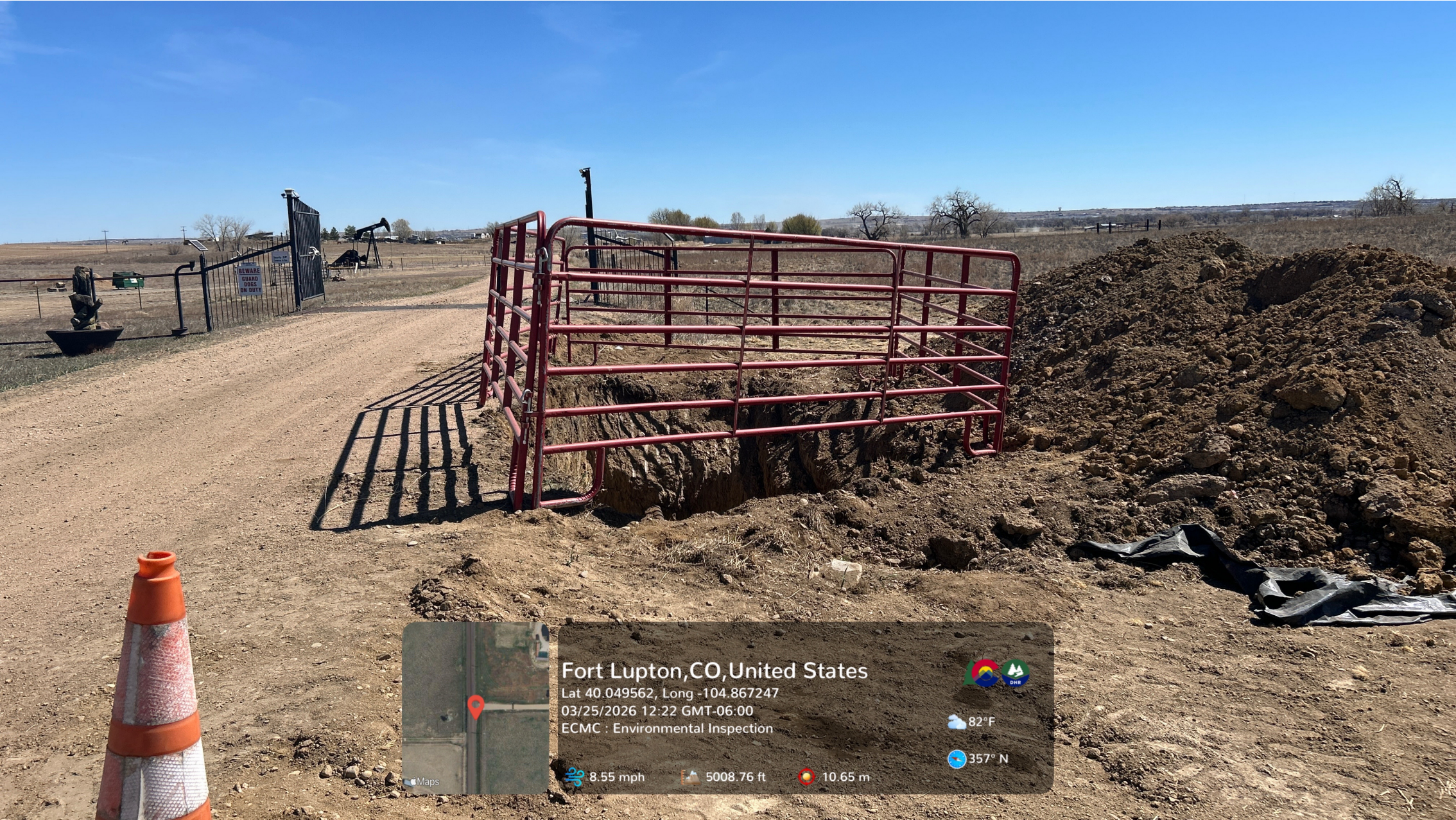
Metal panel fencing surrounds the open excavation. Sign on black metal fence in background reads, " BEWARE GUARD DOGS ON DUTY".
