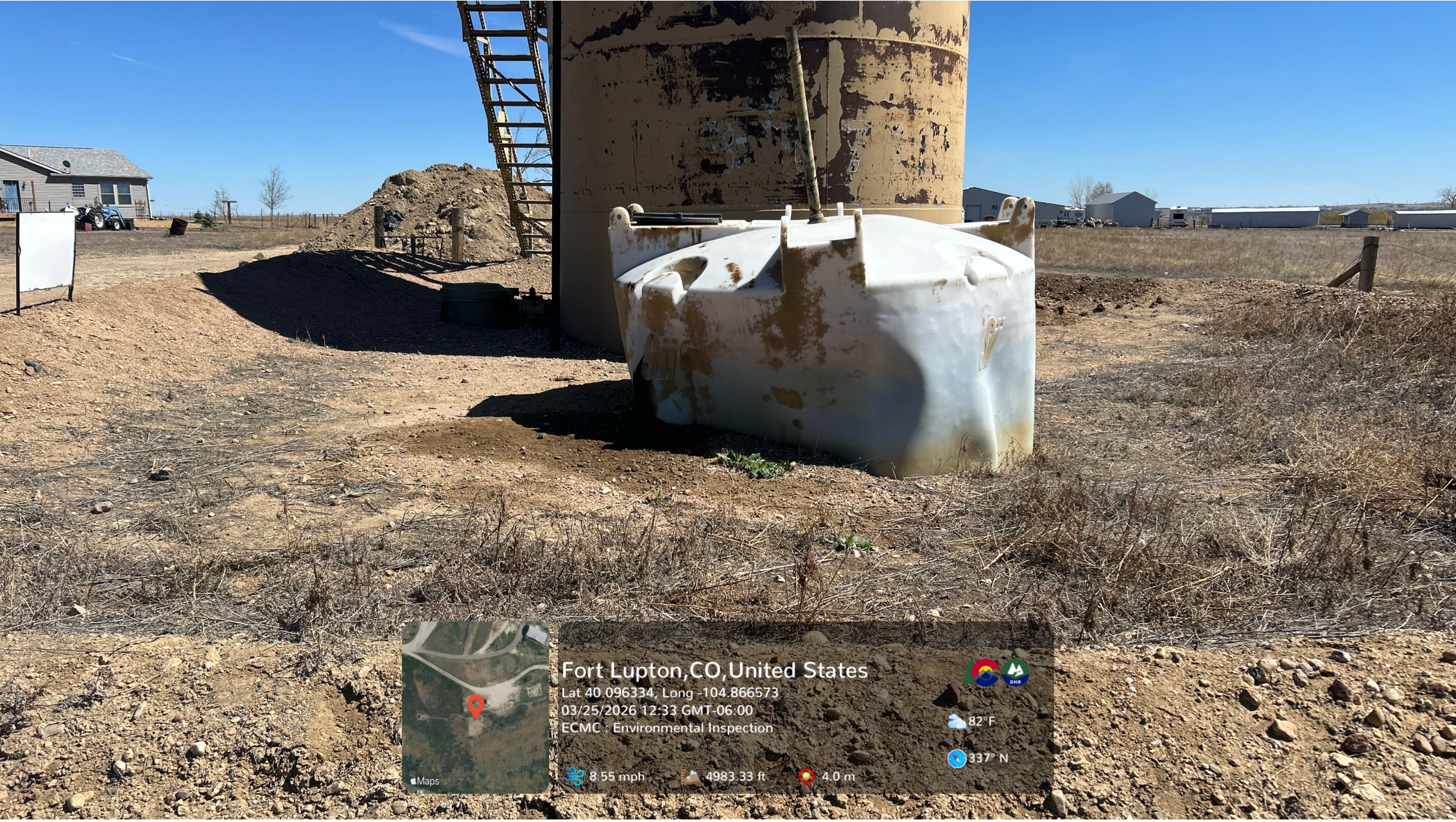
Stained soil is visible beneath a crack in the 50-bbl partially buried polyethylene produced water tank.
