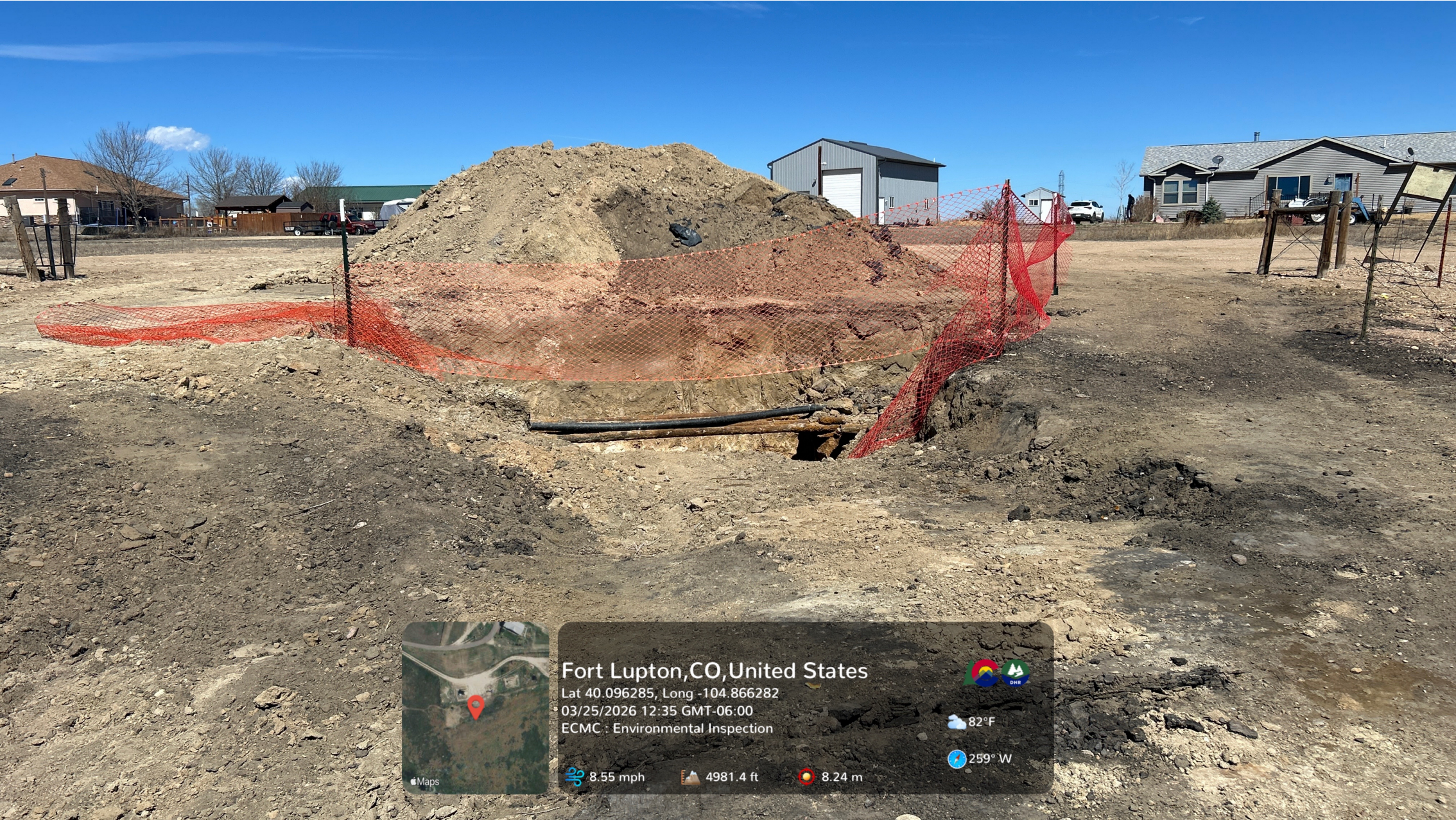
Hydrocarbon stained soil at the surface to the west and south of the excavation.
