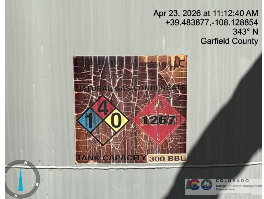
Photo # 2368 Condensate tank label damaged & some required information is illegible
