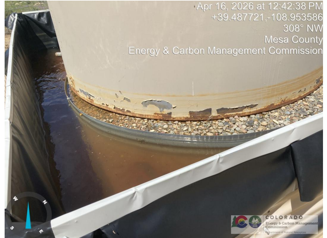
Storm water in tank berm.
