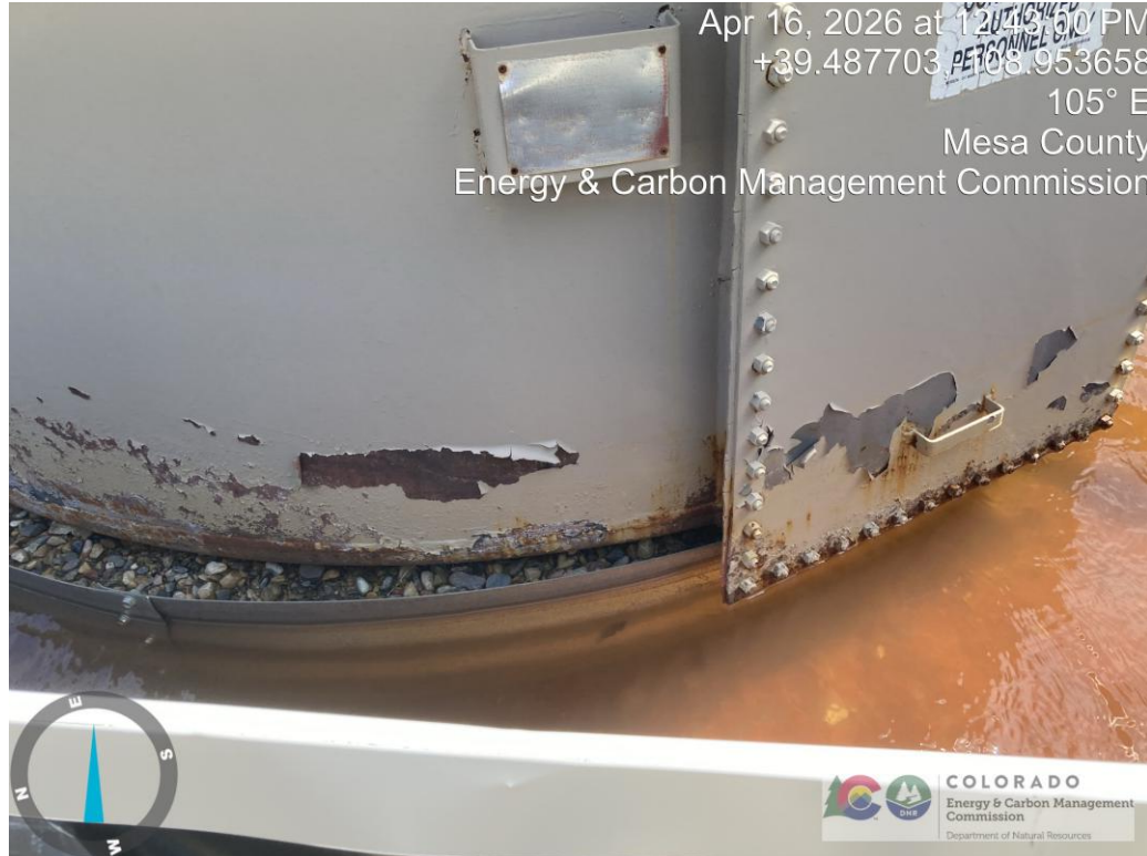
Storm water in tank berm.
