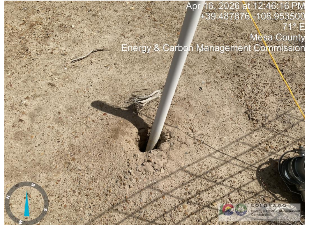
Vent line hole is not in the ground securely.
