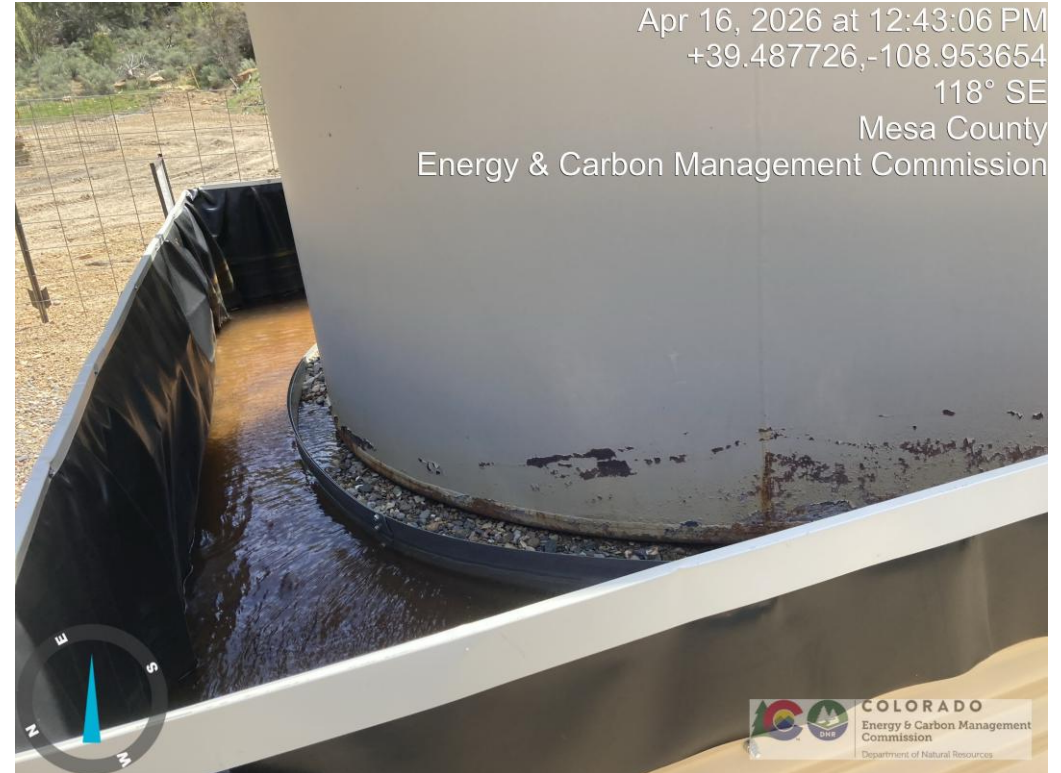
Storm water in tank berm.
