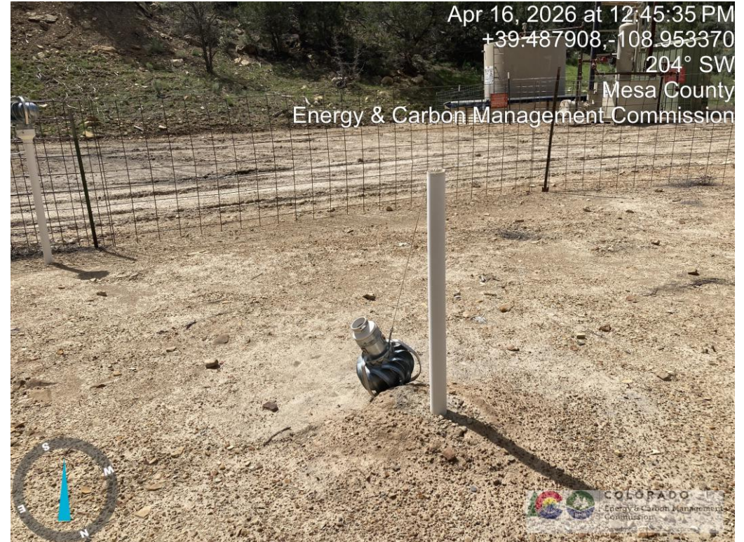
Turbine off of vent.
