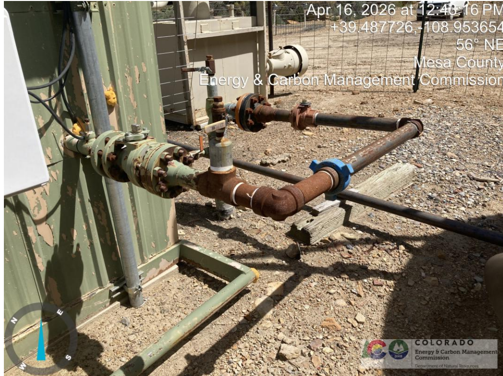
Unpainted rusty lines.
