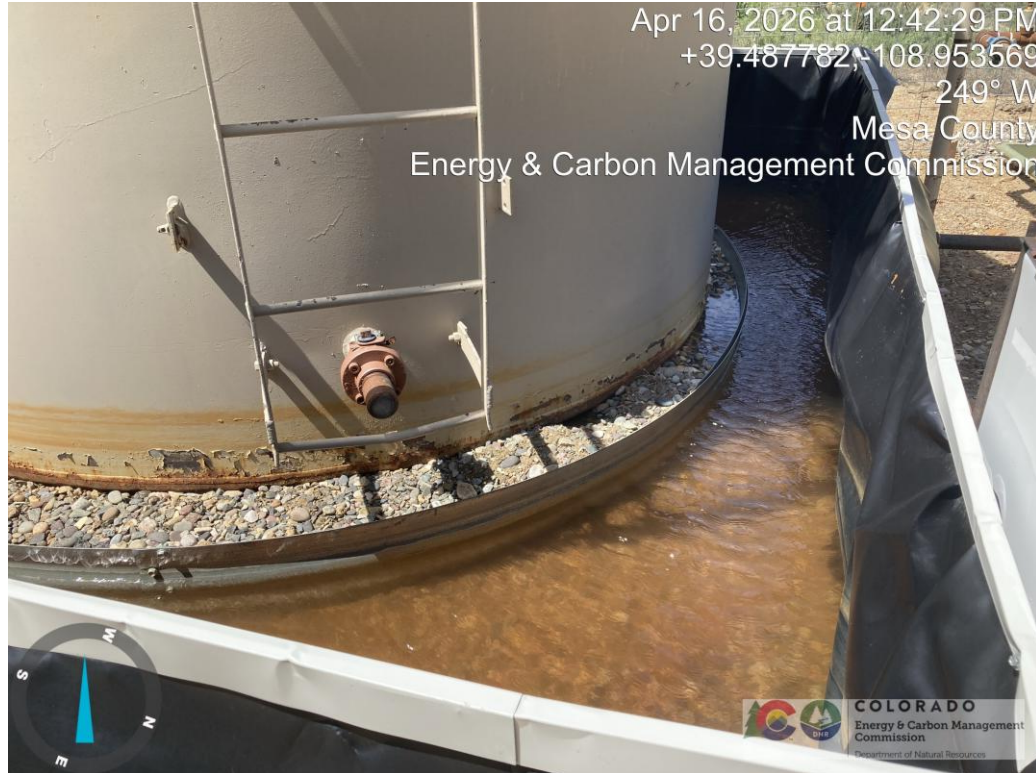
Storm water in tank berm.
