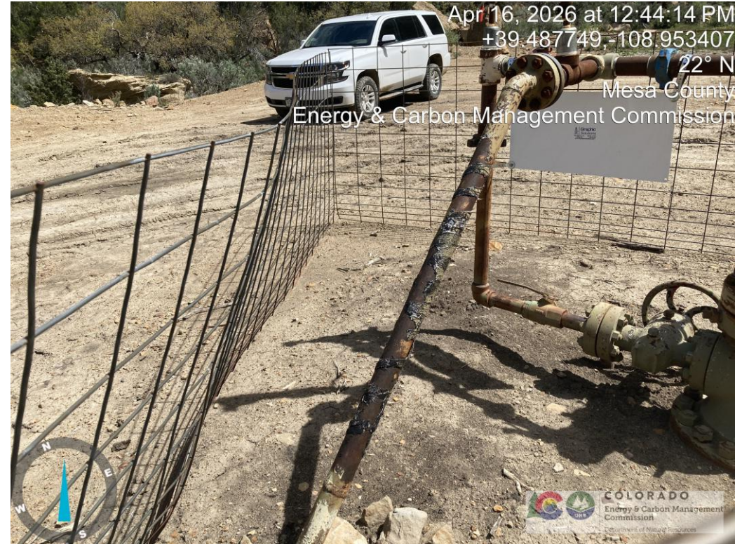
Riser line has coating material damage.
