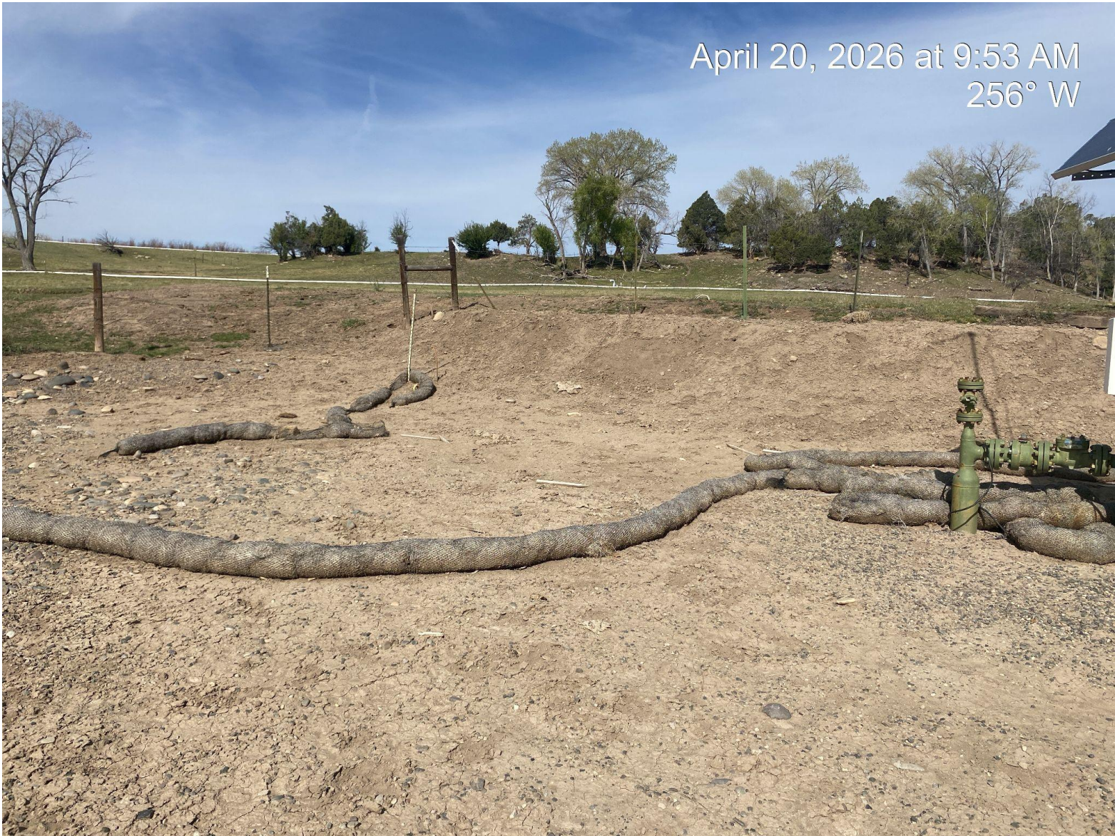
Photo 2. Wattles installed are no longer functioning.
