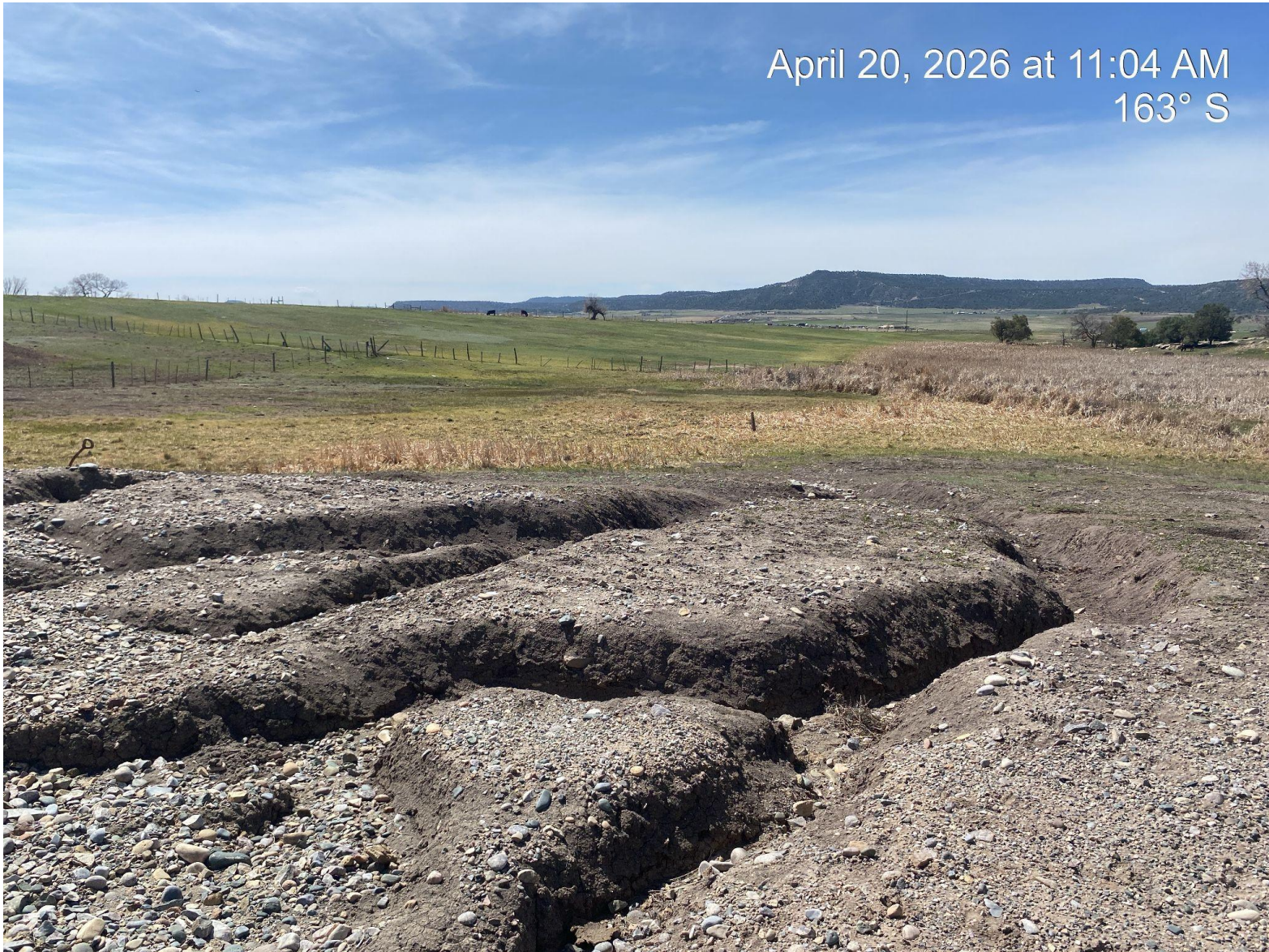
Photo 2. View of deep gully erosion persisting on the southern edge of the pad.
