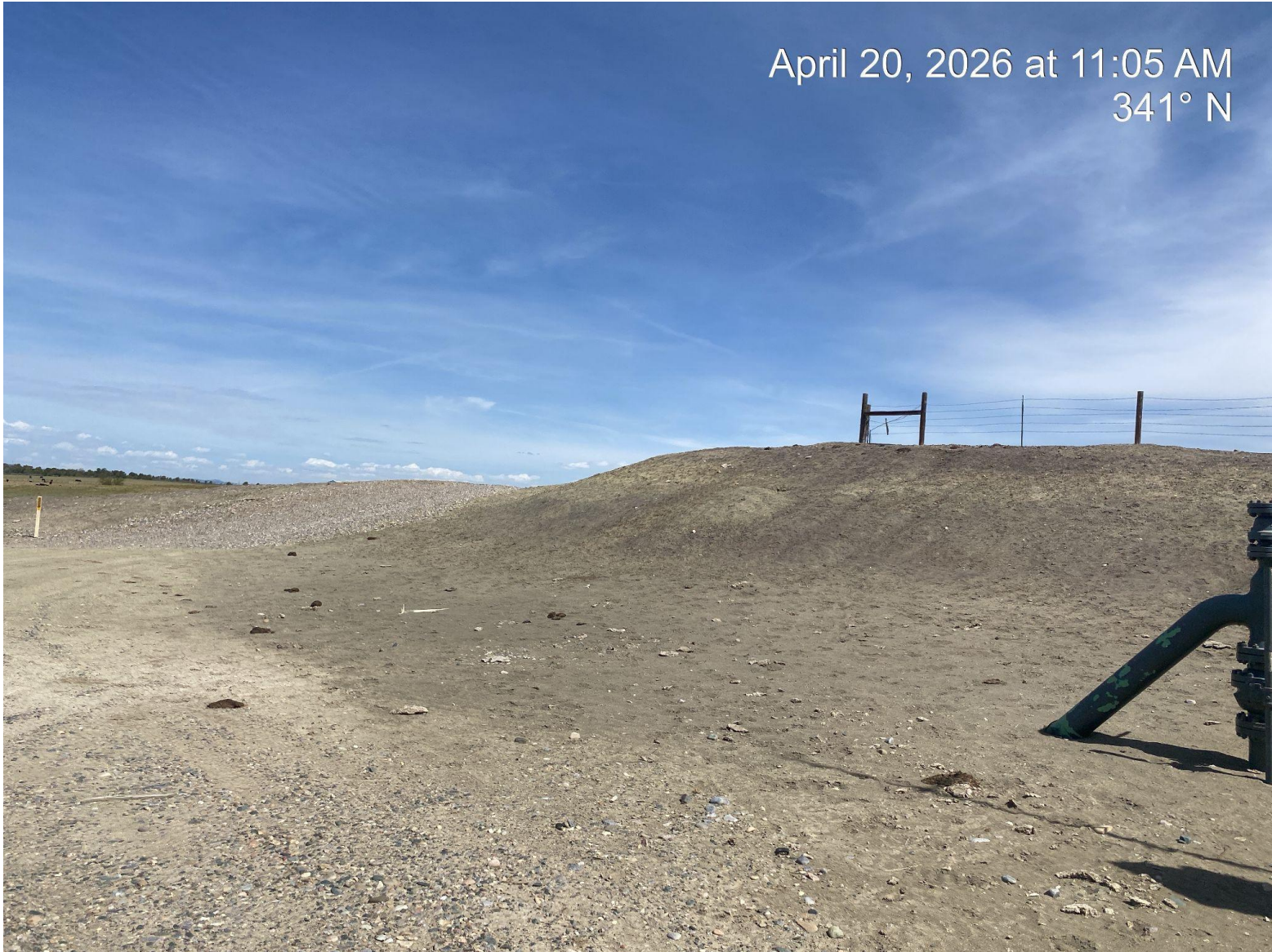
Photo 3. View of location cutslope which remains with minimal vegetation and bare loose soils.
