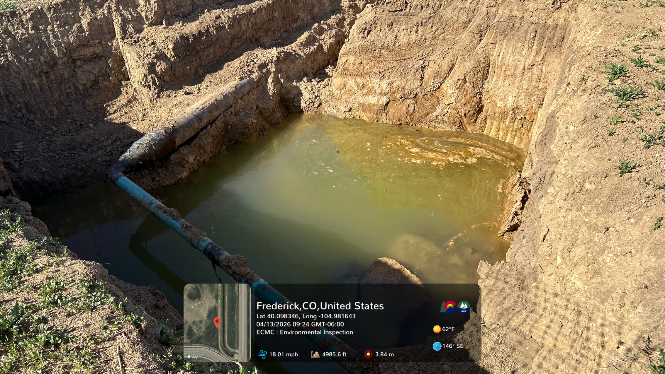
Stained soil and groundwater with free product are visible in situ.
