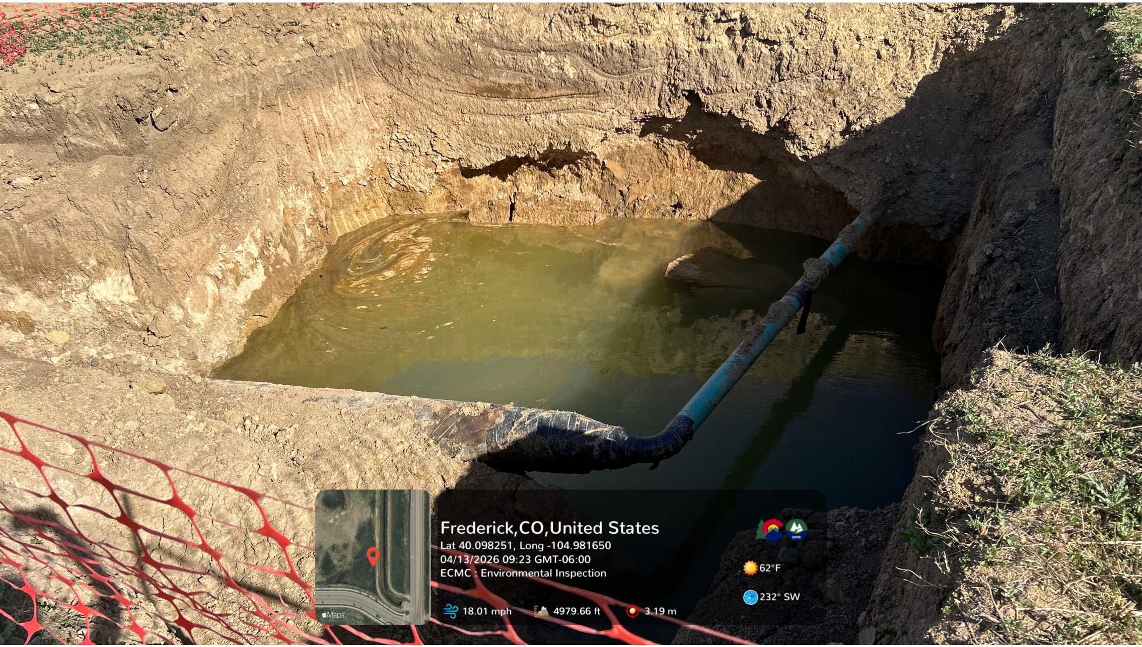
Stained soil and groundwater with free product are visible in situ. Soil mass failures are visible on the excavation sidewalls.
