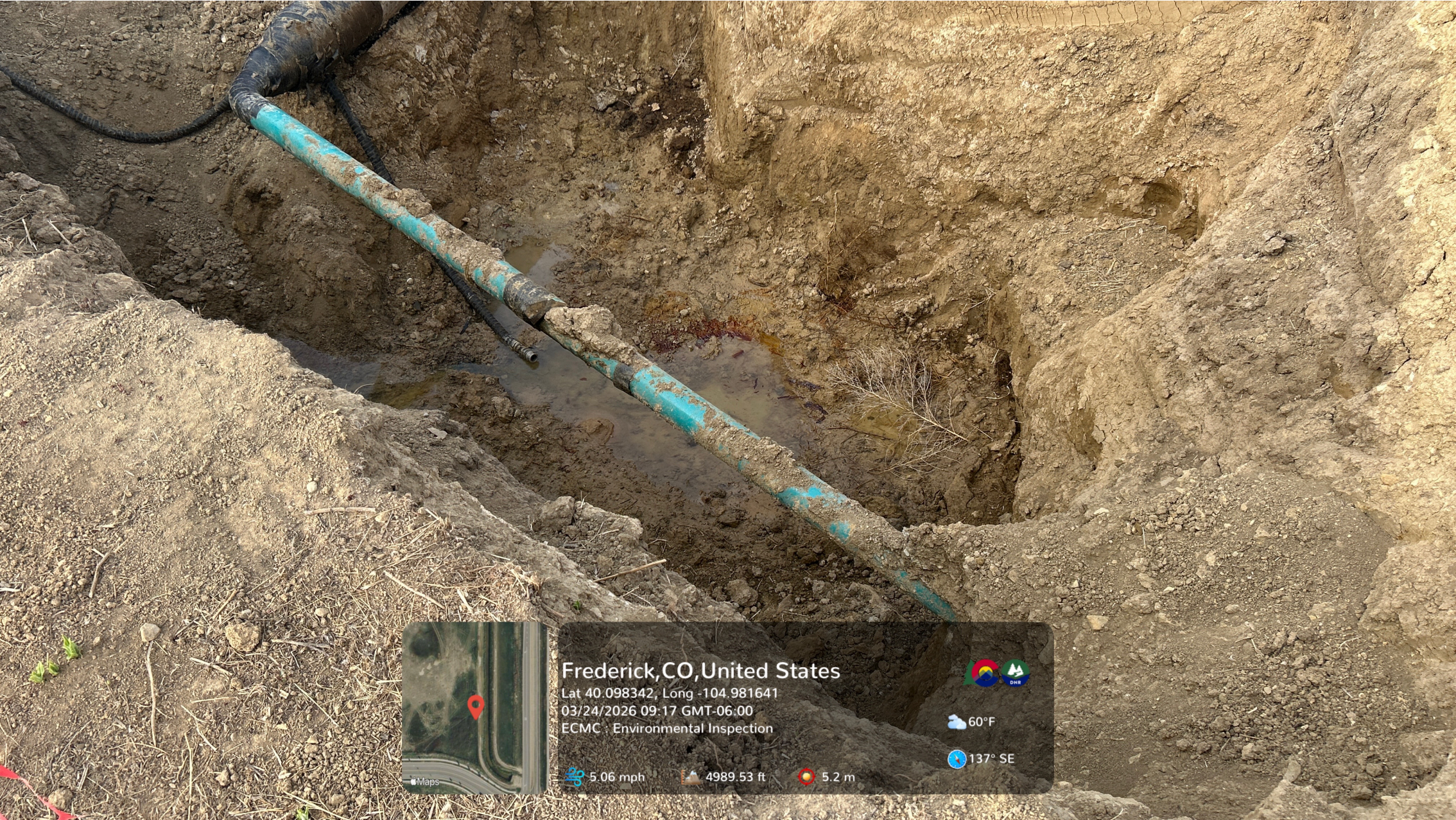
Stained soil is visible in situ.
