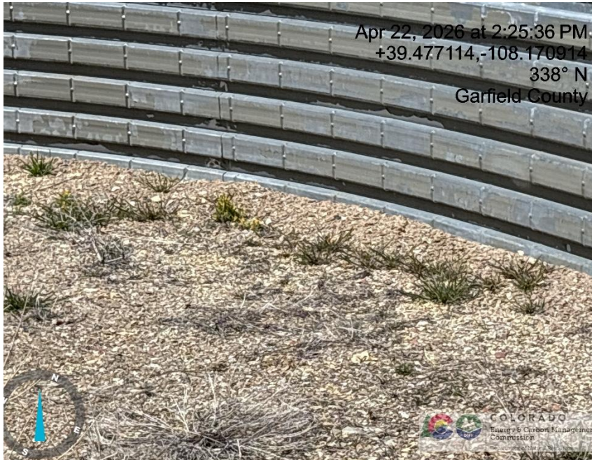
Photo # 2035 Weeds in secondary containment
