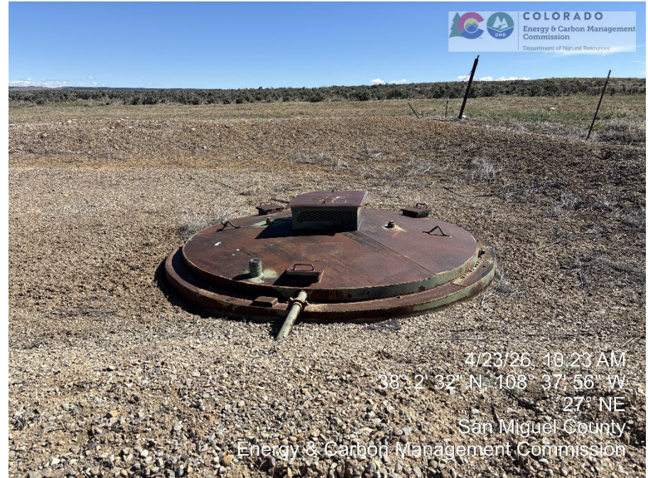
Tank with no labels
