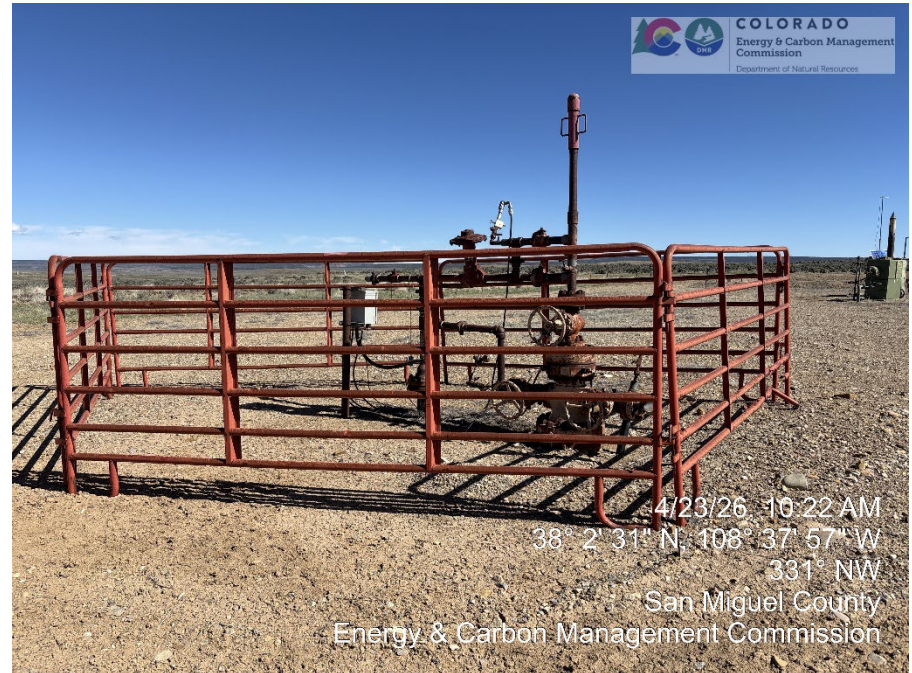
Wellhead with fence
