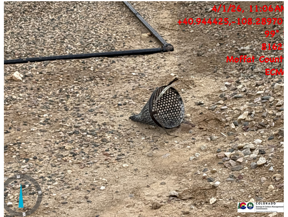
Bird protector for heater on condensate tank
