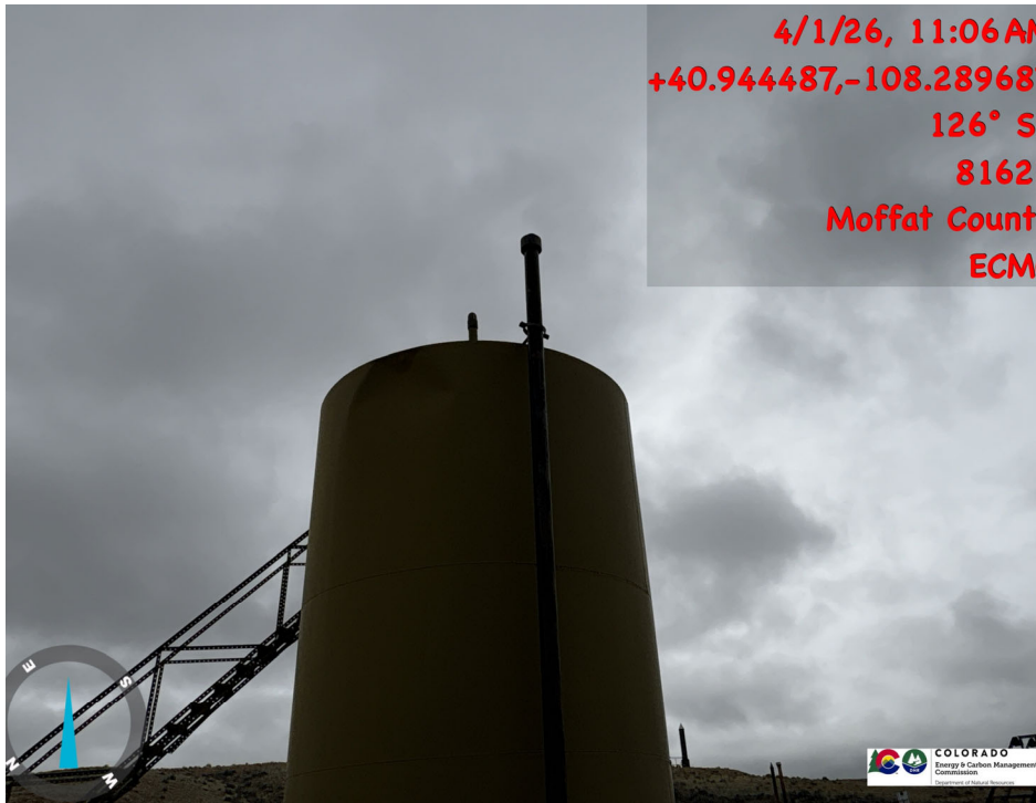
Bird protector missing
