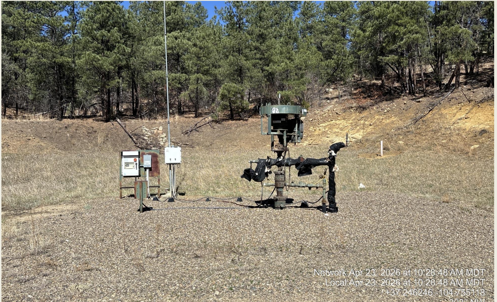
PHOTO 4: ORIG. WELLHEAD AND EQUIPMENT.
