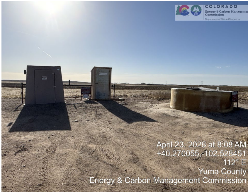
Meter run and Tank
