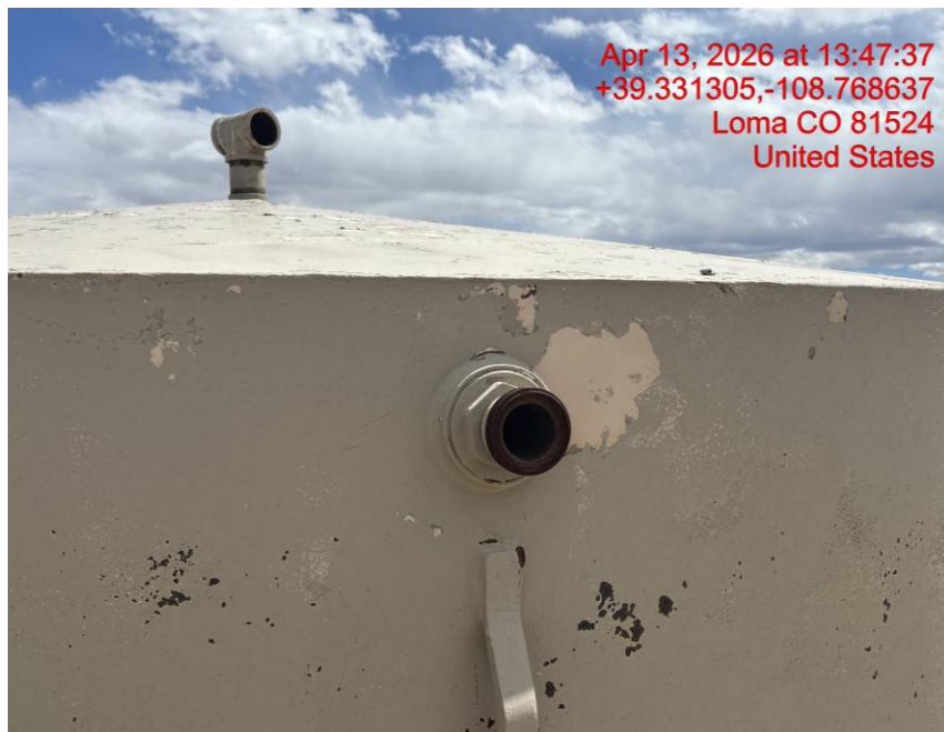
Wildlife Entry Hazards – Photo #03529
