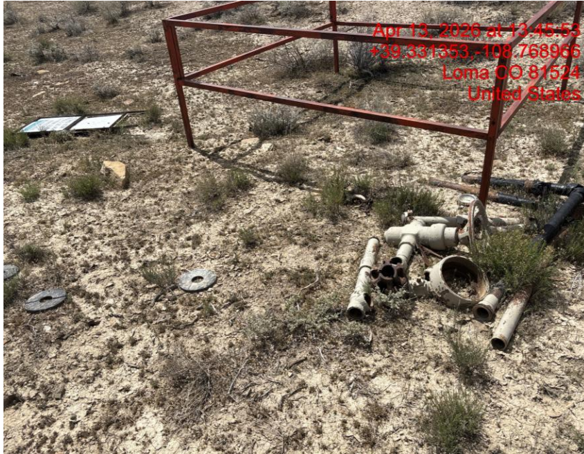
Wellhead Fencing/Debris – Photo #03519
