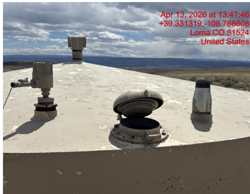
Wildlife Entry Hazard – Photo #03530
