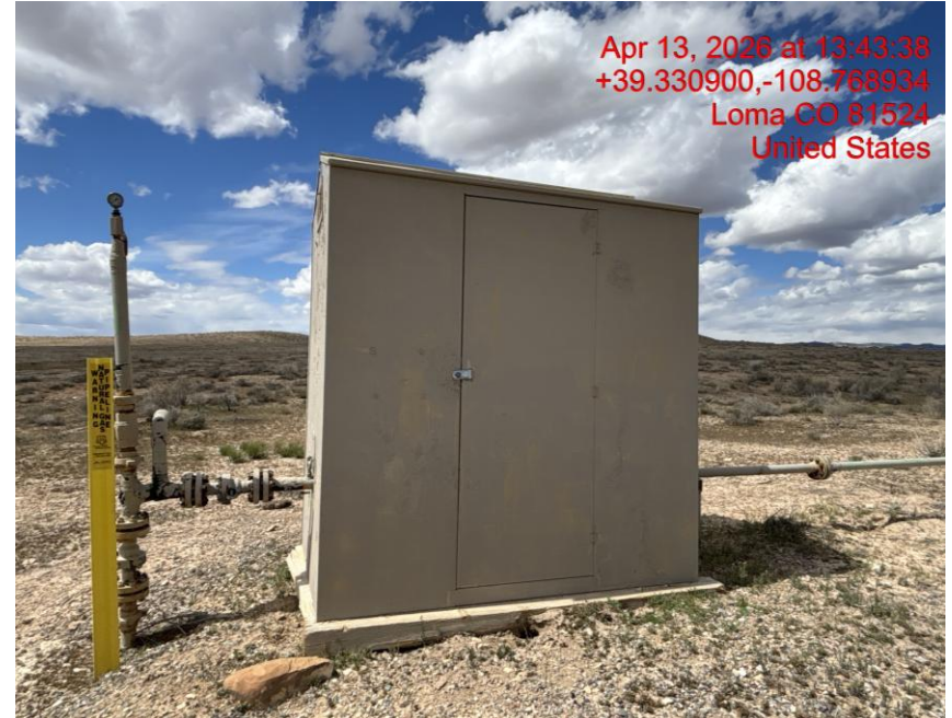
Unused Gas Meter – Photo #03513
