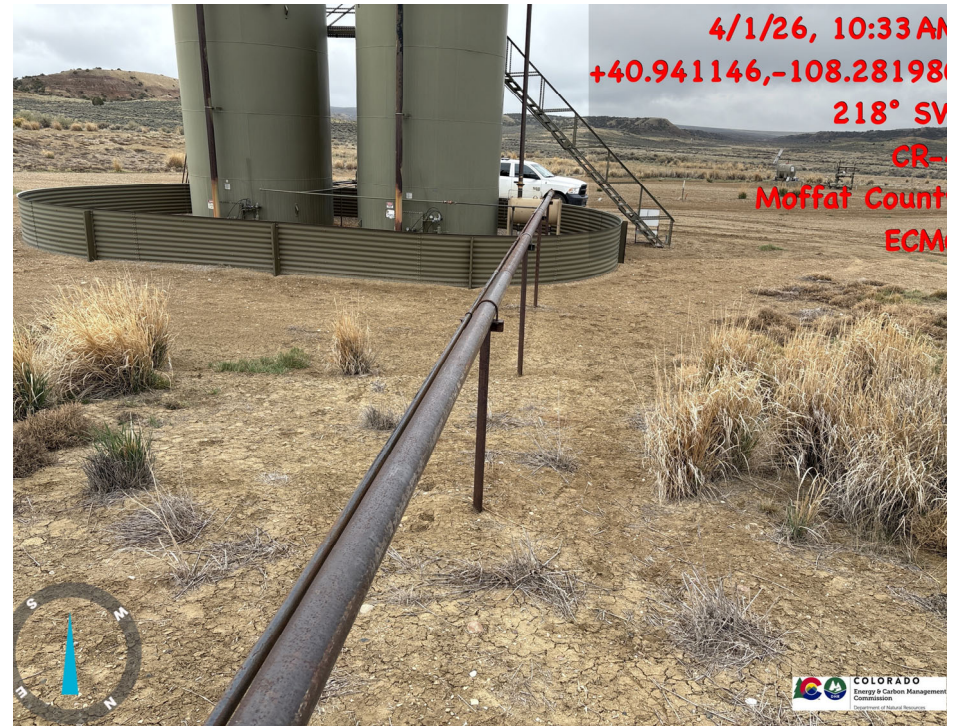
Line for ECD from tanks
