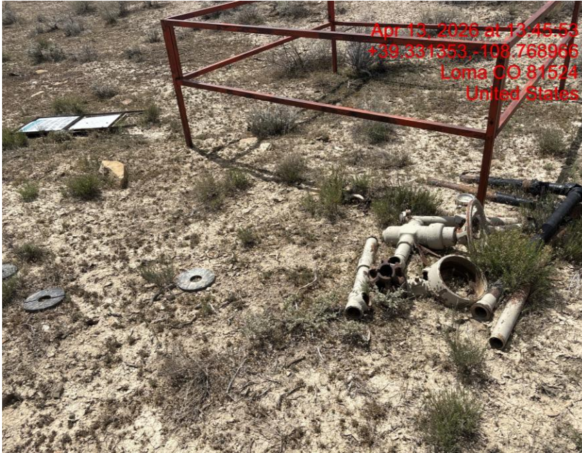
Wellhead Fencing/Debris – Photo #03519
