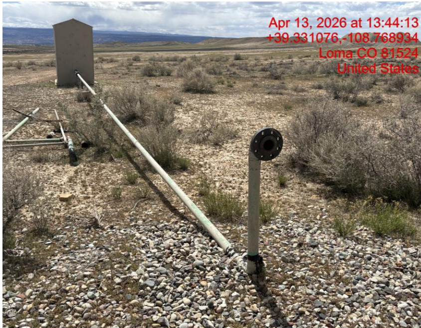
Unused Gas Meter – Photo #03515
