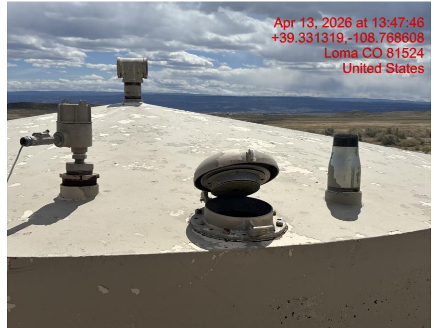
Wildlife Entry Hazard – Photo #03530
