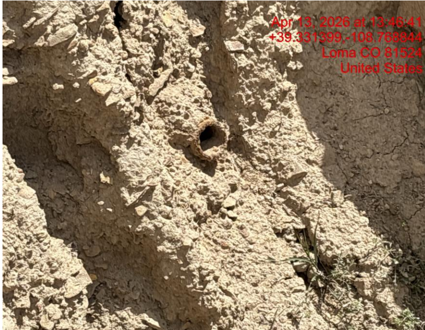
Open-Ended Flowline – Photo #03523
