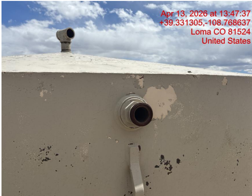
Wildlife Entry Hazard – Photo #03529
