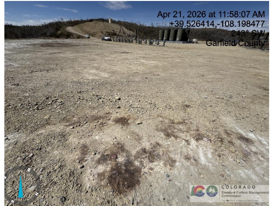
Photo # 1406 Staining on location
