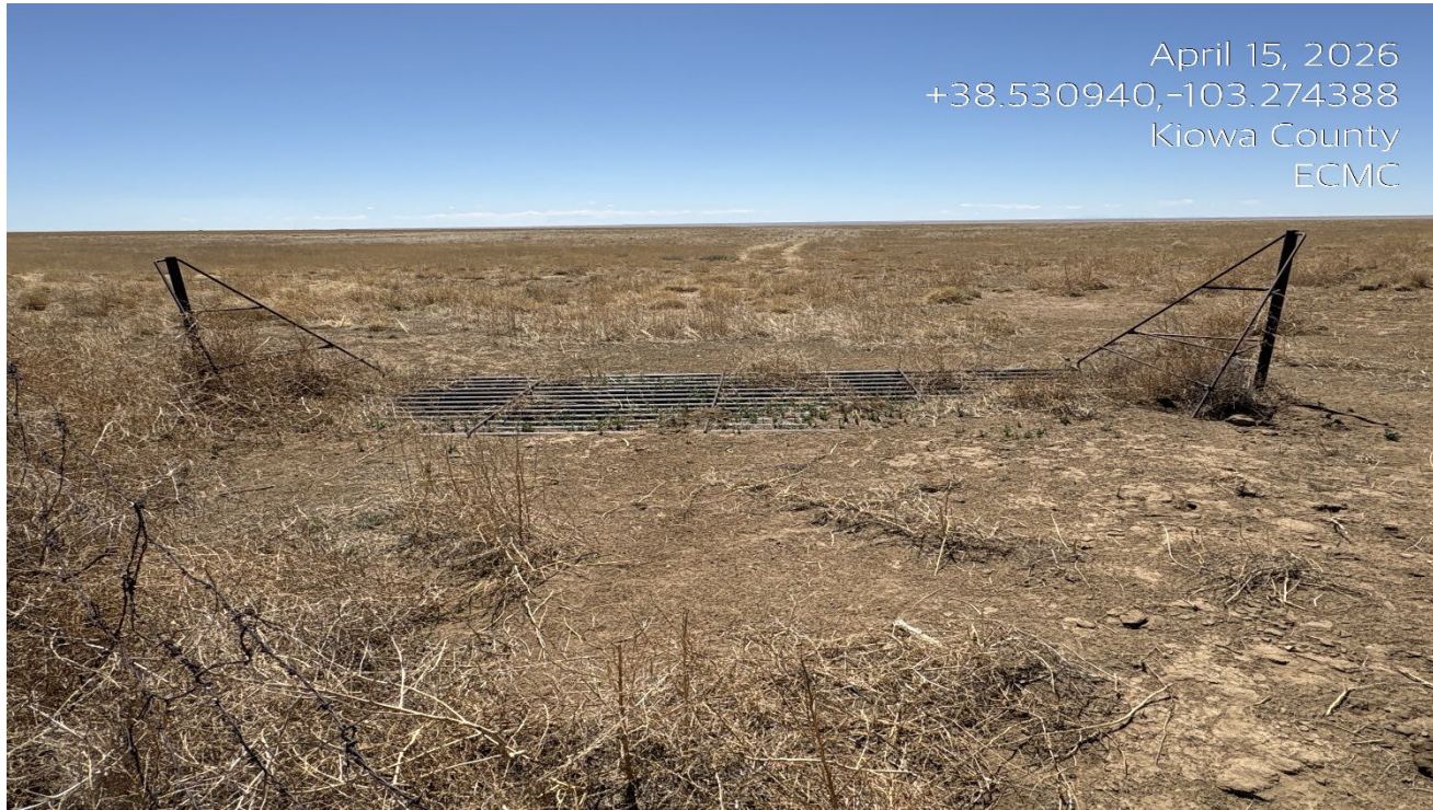
Photo 1. Facing southwest at the beginning of the access road. The cattle guard was never removed and is not attached to the fence line.
