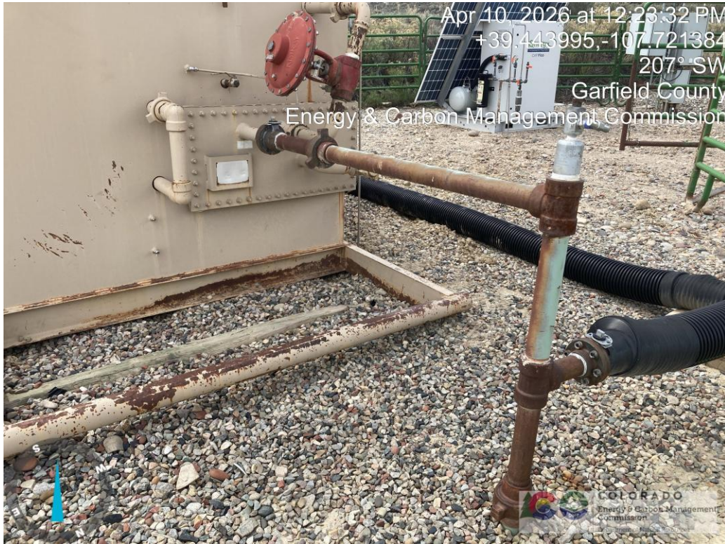
Unpainted flowlines and paint deterioration with areas of rust.
