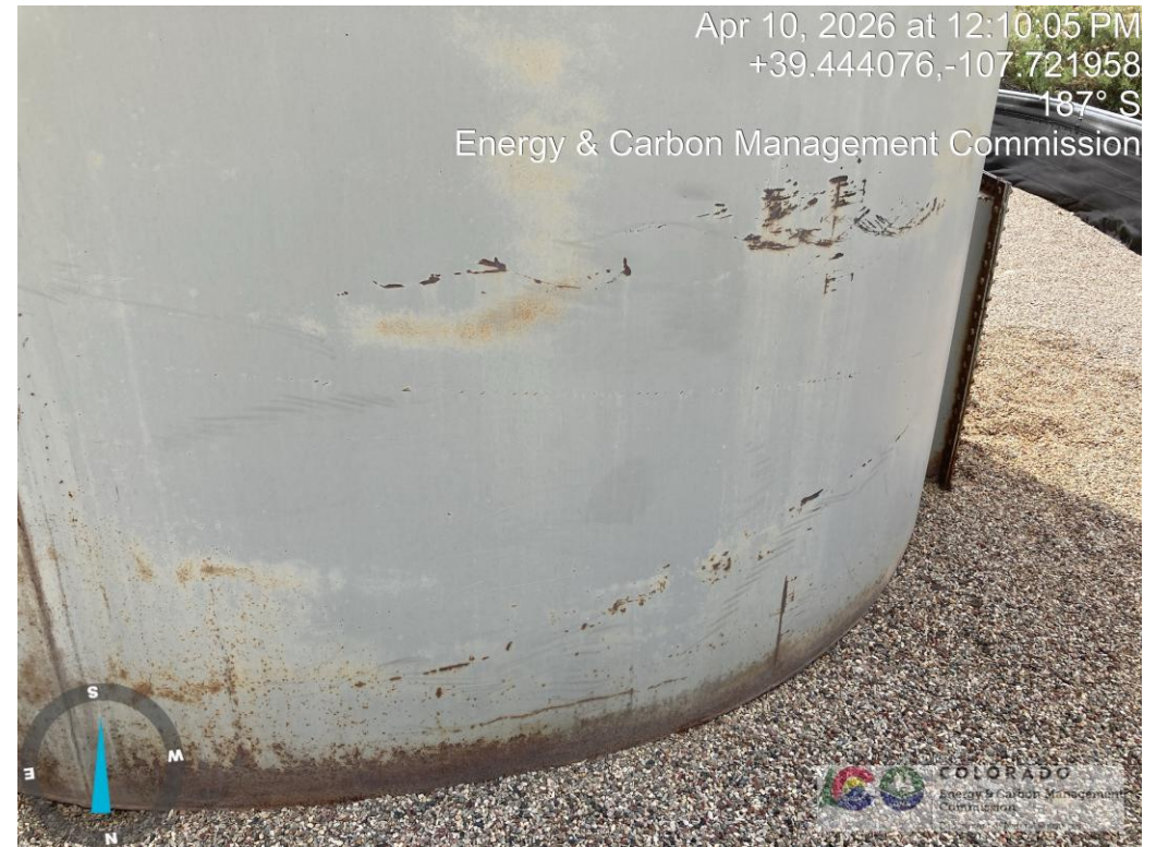
Paint deterioration and areas of rust.
