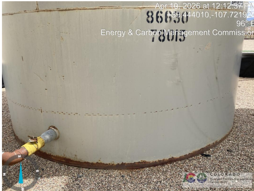
Paint deterioration and areas of rust.
