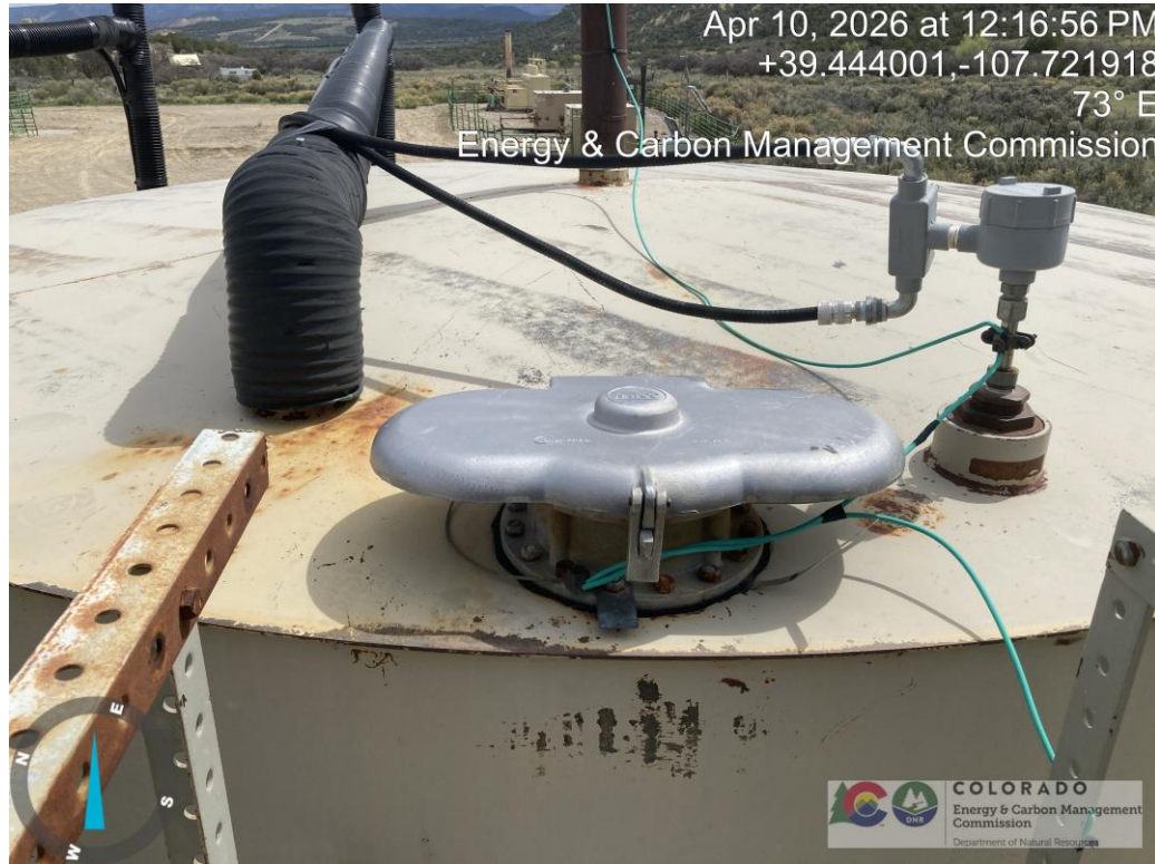
Top of tank is rusted out around the dumphline inlet.
