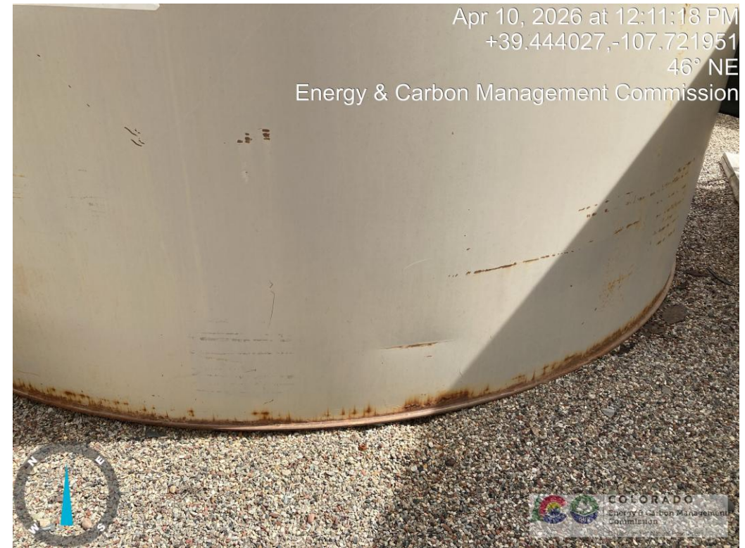
Paint deterioration and areas of rust.
