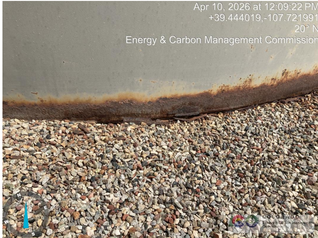
Paint deterioration and areas of rust.
