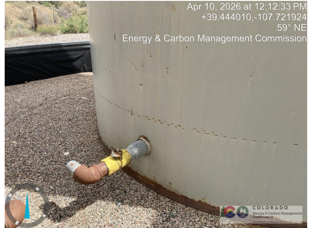
Paint deterioration and areas of rust.
