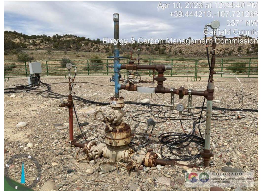
Unpainted and paint deterioration of flowlines and well head equipment with areas of rust.
