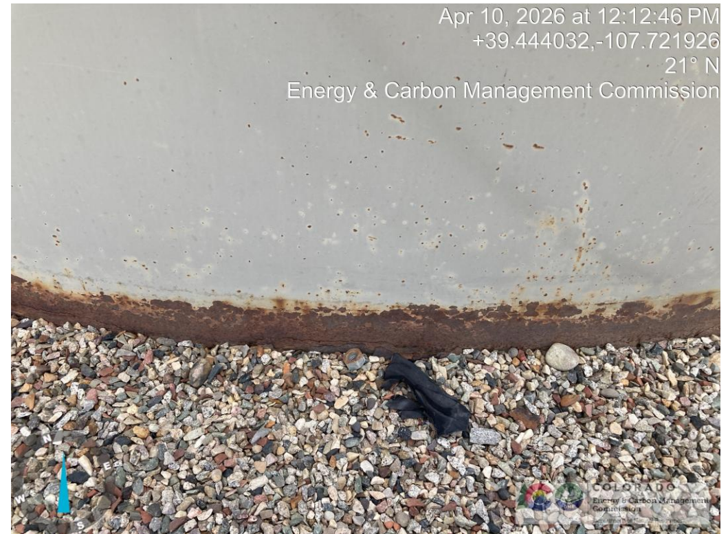
Paint deterioration and areas of rust.
