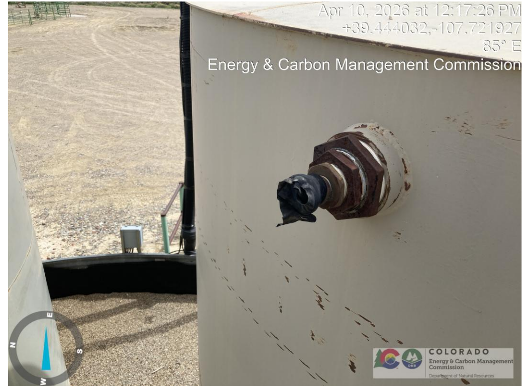
Rusted and tapped inlet fittings
