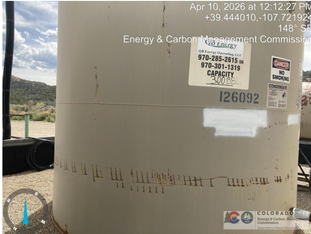
Paint deterioration and areas of rust.
