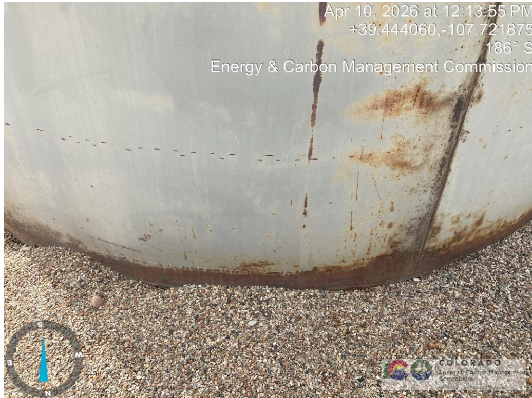
Paint deterioration and areas of rust.
