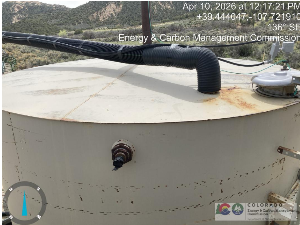
Top of tank is rusted out around the dumlaine inlet.
