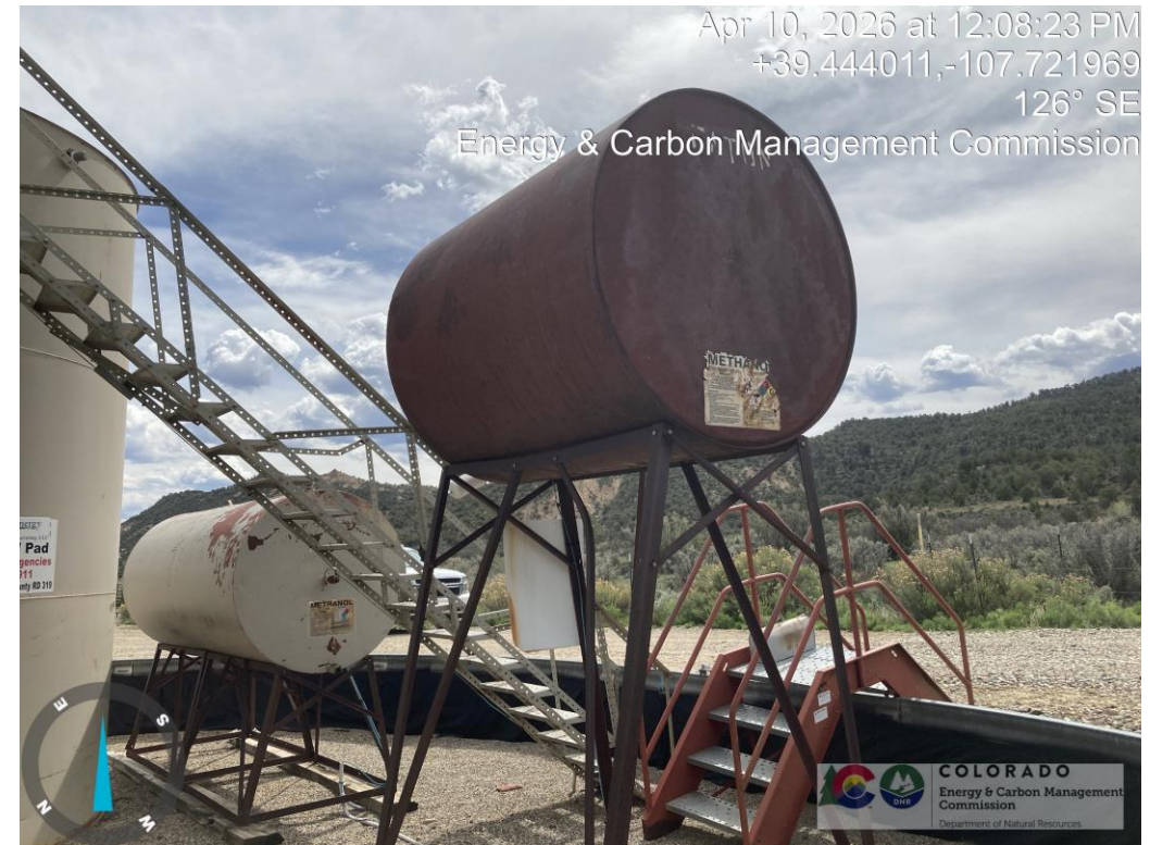
Methanol tank paint is in poor condition or lacks paint. Label is in poor condition.
