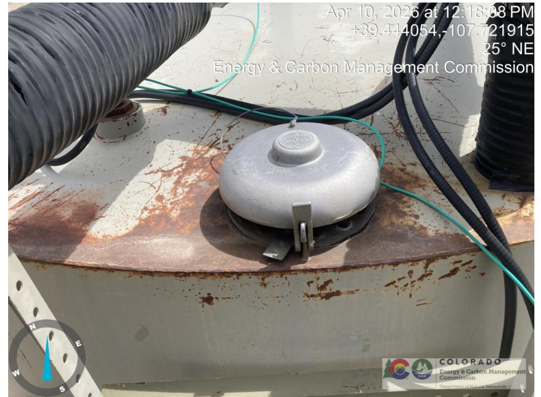
Paint deterioration and areas of rust.
