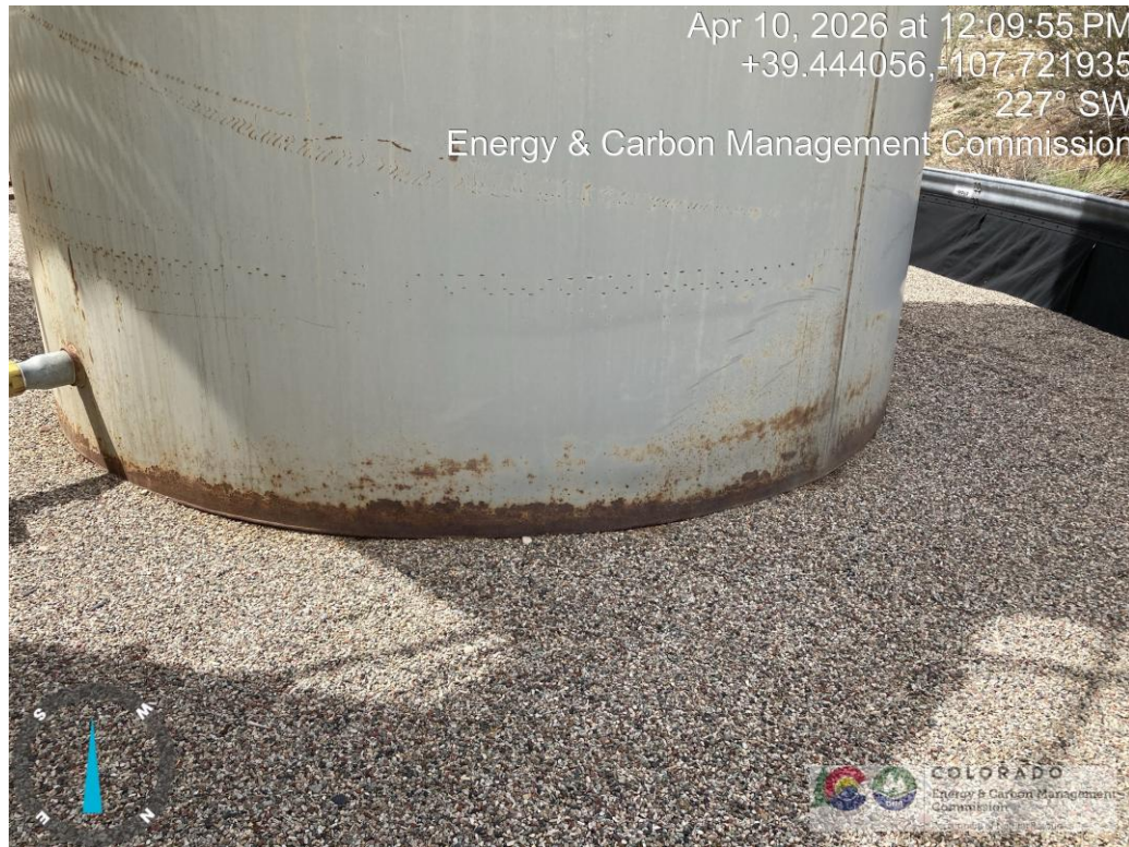
Paint deterioration and areas of rust.
