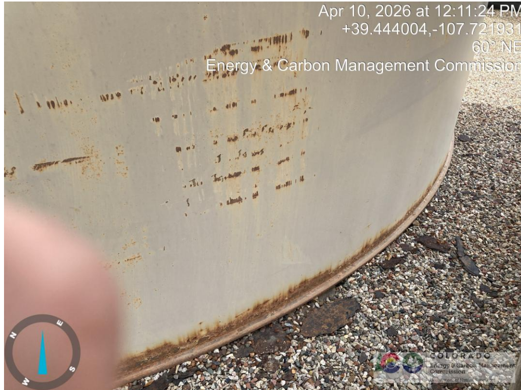
Paint deterioration and areas of rust.
