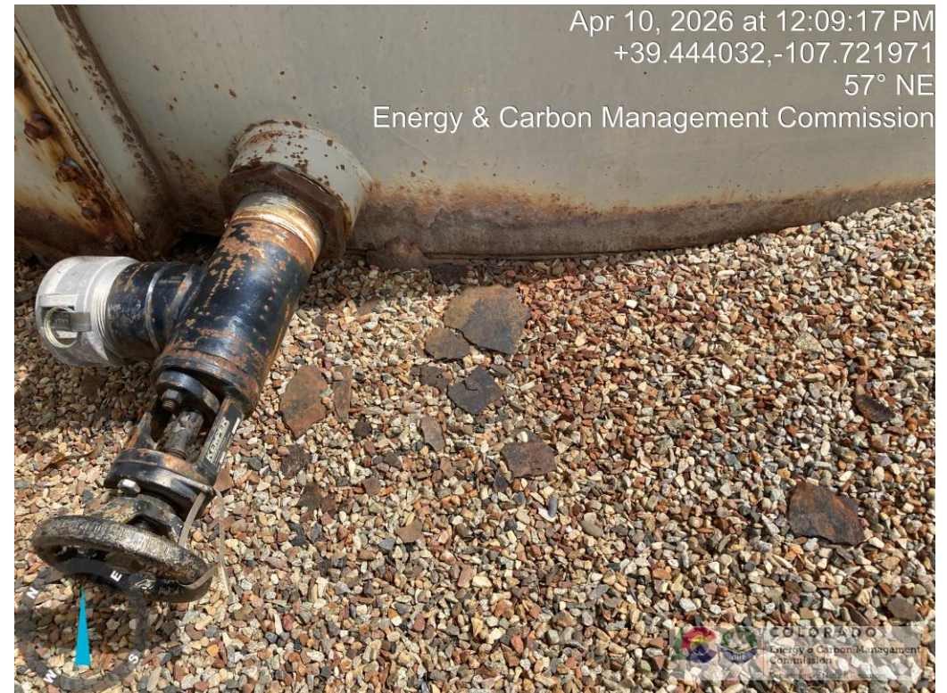
Paint deterioration and areas of rust.
