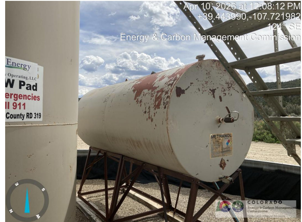
Methanol tank paint is in poor condition.
