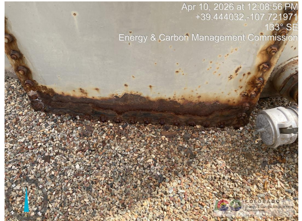
Rusted and flaking tank man hatch.
