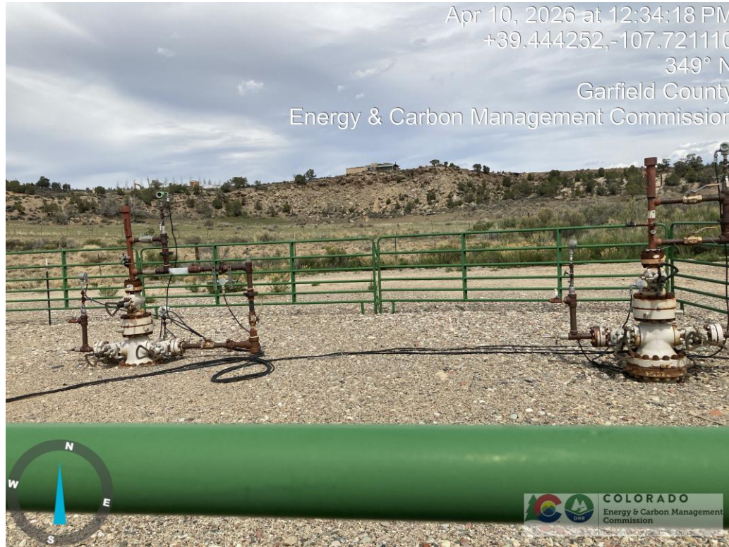
Unpainted and paint deterioration of flowlines and well head equipment with areas of rust.
