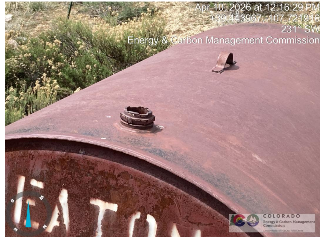
No lid on top of methanol tank.
