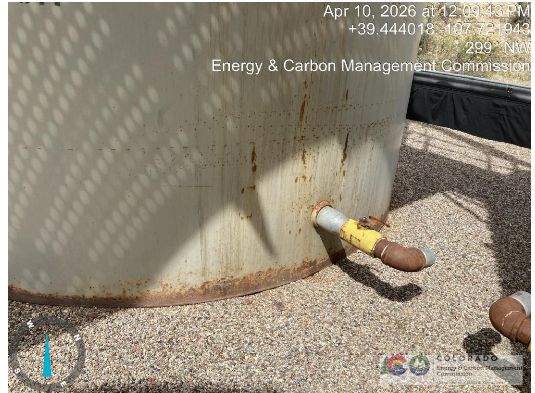
Paint deterioration and areas of rust.
