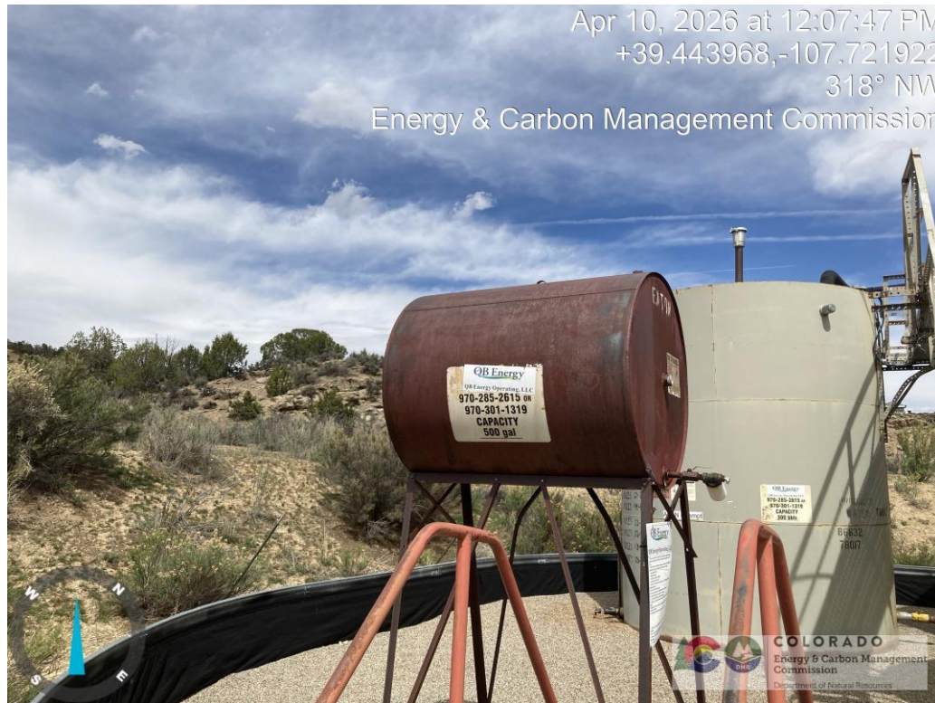
Methanol tank paint is in poor condition or lacks paint.
