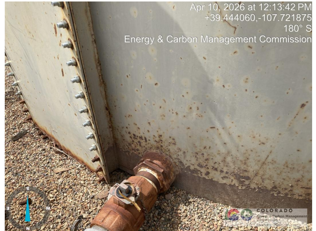
Paint deterioration and areas of rust.
