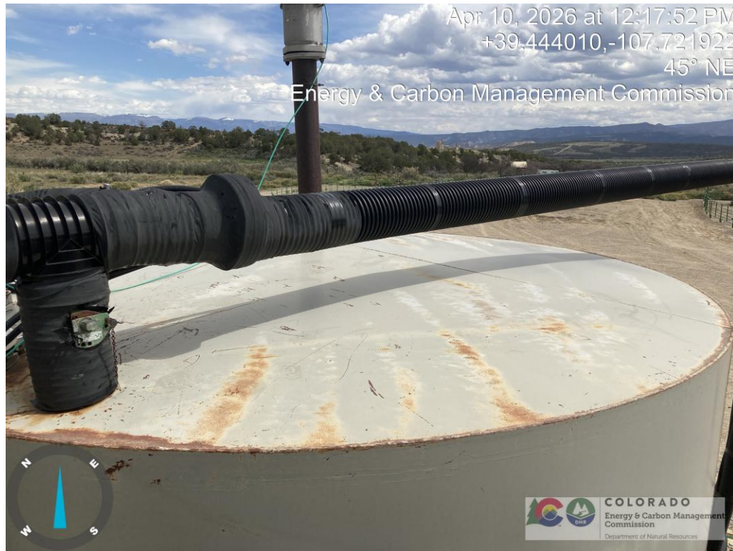
Paint deterioration and areas of rust.
