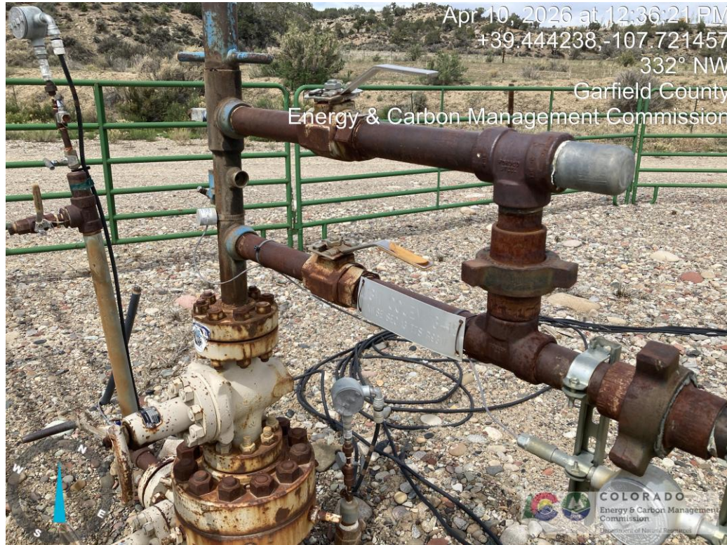
Unpainted and paint deterioration of flowlines and well head equipment with areas of rust.
