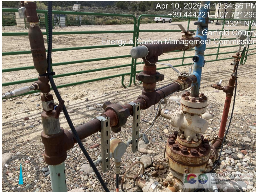
Unpainted and paint deterioration of flowlines and well head equipment with areas of rust.
