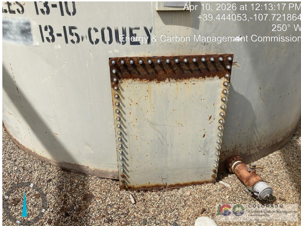
Rusted and flaking tank man hatch and bolts.
