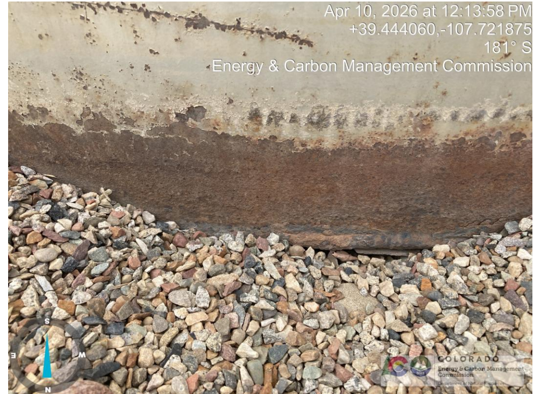
Paint deterioration and areas of rust.
