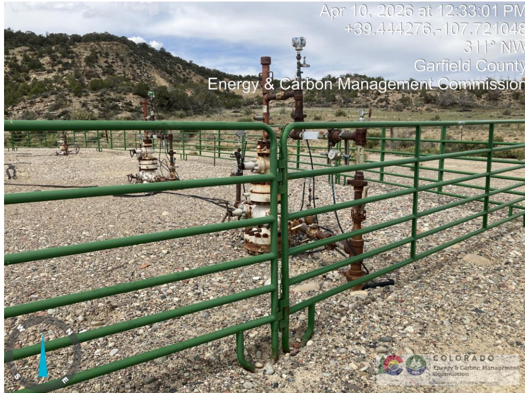
Unpainted and paint deterioration of flowlines and well head equipment with areas of rust.
