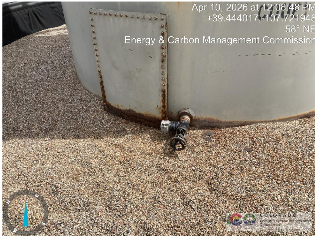
Rust around tank bottoms.
