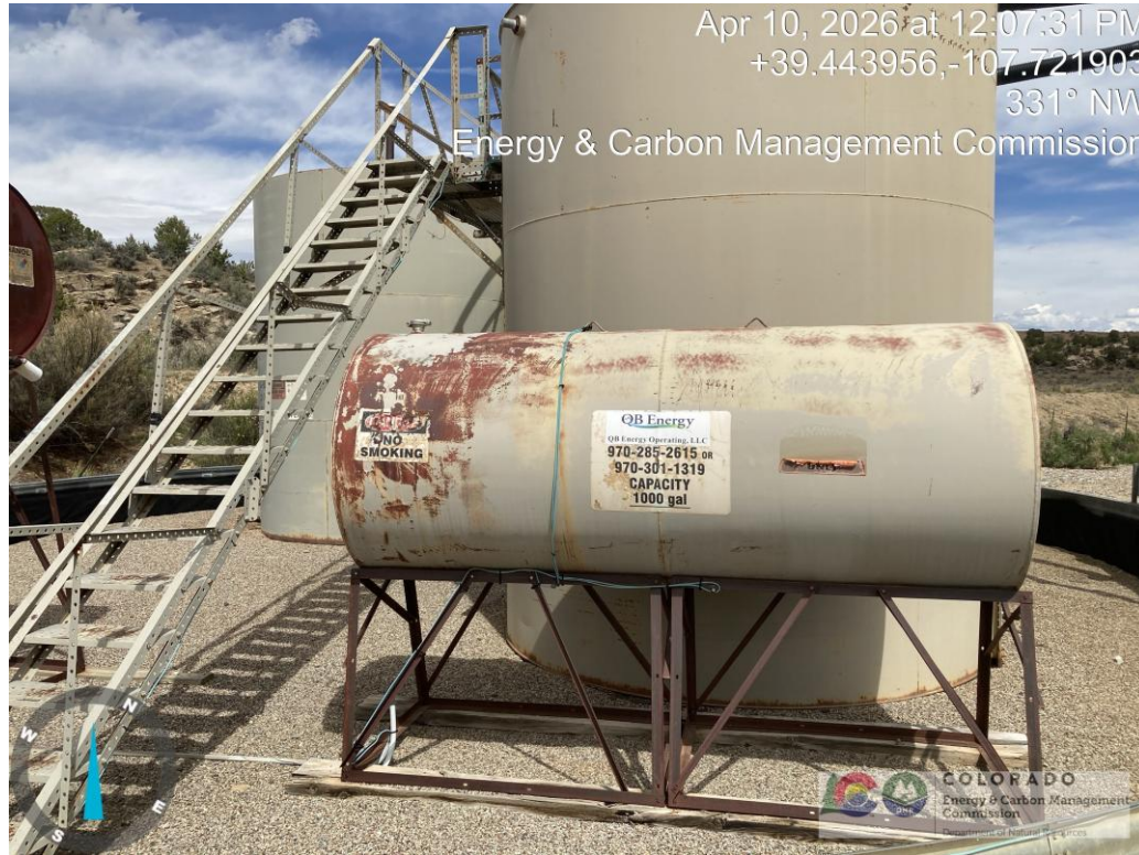
Methanol tank paint is in poor condition, and no smoking sign is in poor condition.
