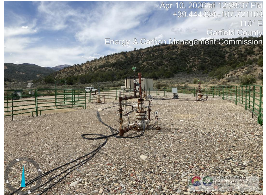
Unpainted and paint deterioration of flowlines and well head equipment with areas of rust.
