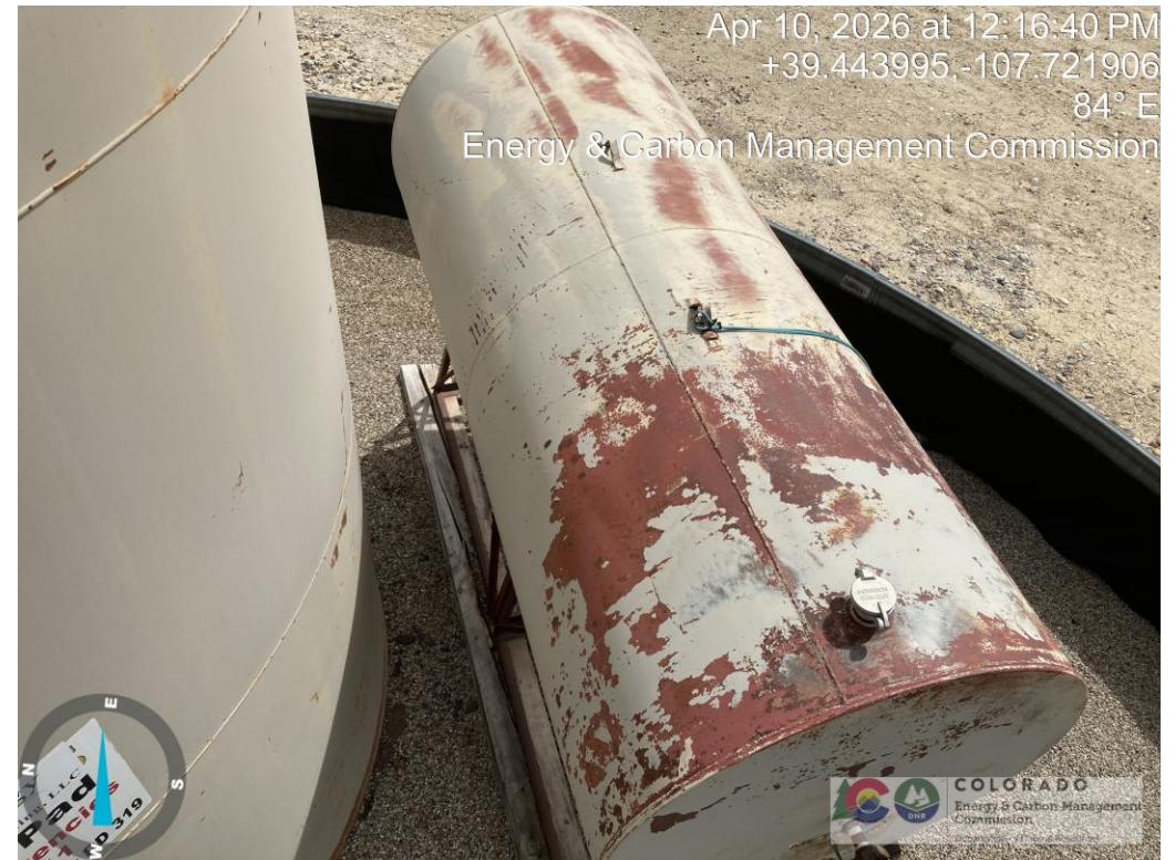
Paint is in poor condition.
