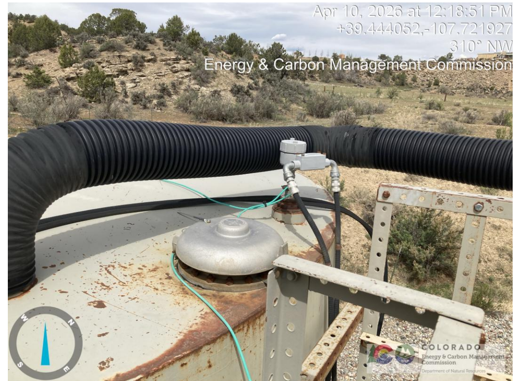
Paint deterioration and areas of rust.
