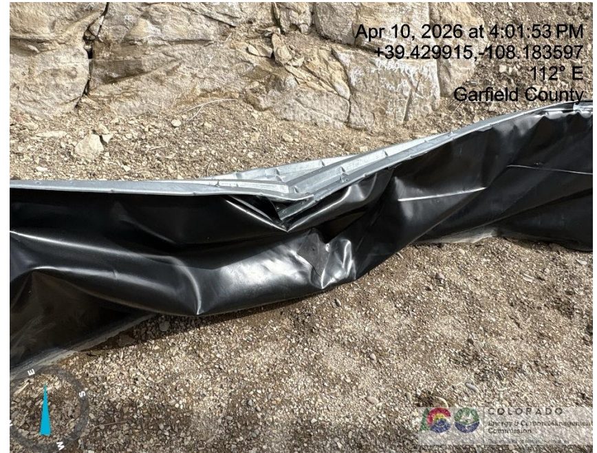
Photo # 8447 Damage to secondary containment
