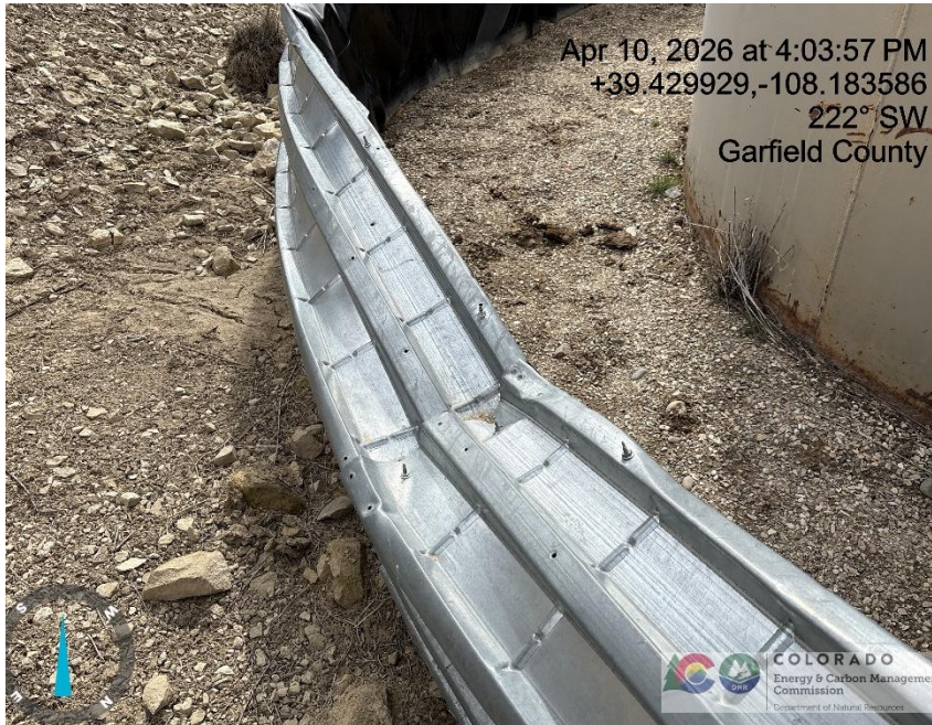
Photo # 8448 Damage to secondary containment
