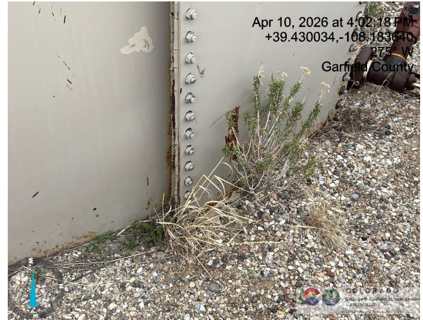
Photo # 8445 Weeds in secondary containment
