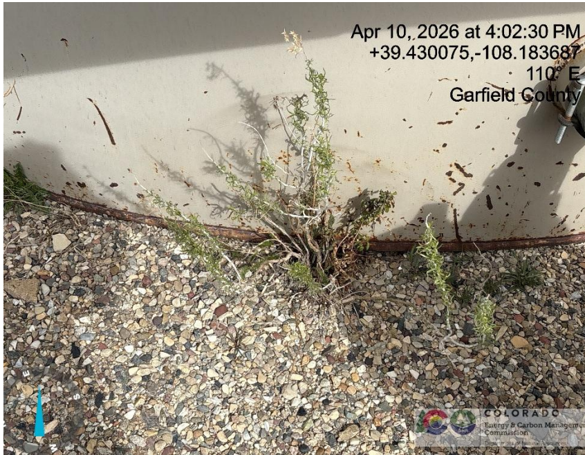
Photo # 8444 Weeds in secondary containment
