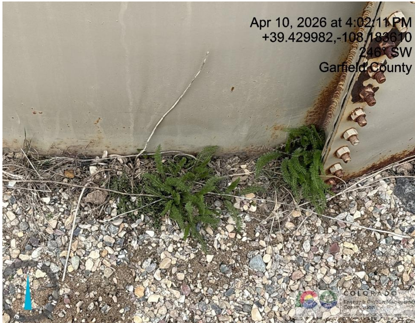
Photo # 8446 Weeds in secondary containment
