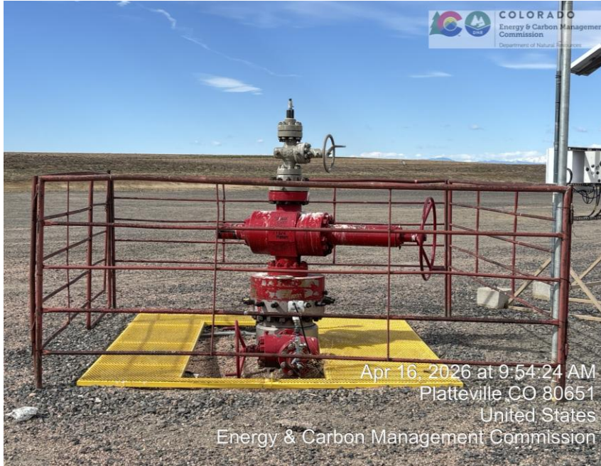
Photo 1 well head and equipment
