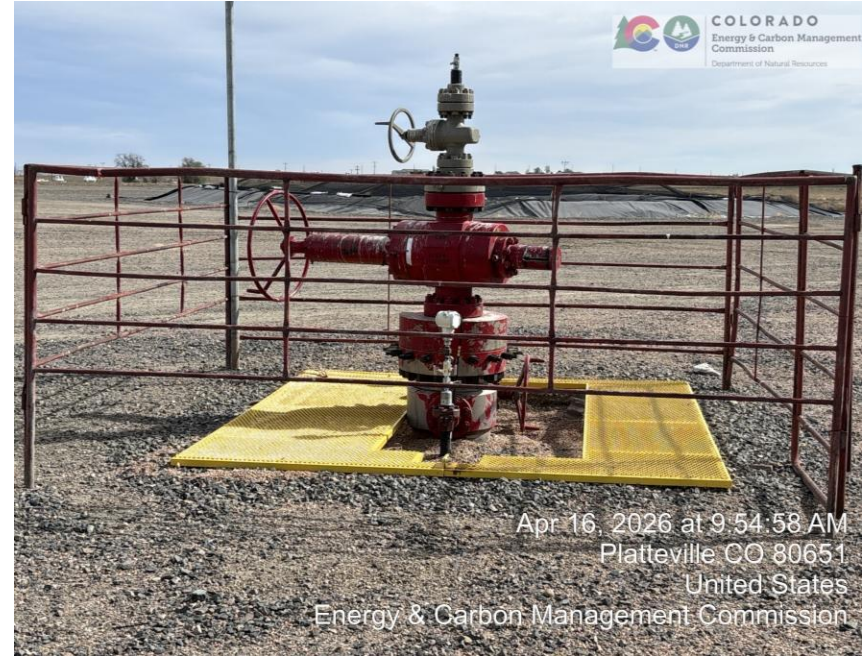
Photo 2 well head and equipment
