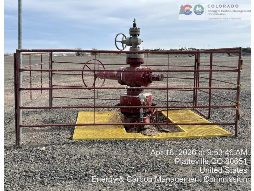
Photo 2 well head and equipment
