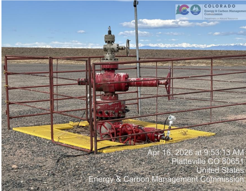
Photo 1 well head and equipment
